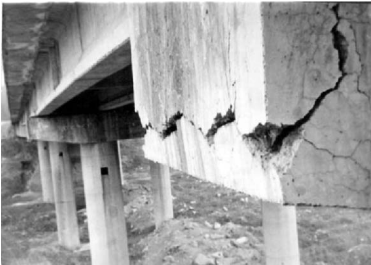
Figure 2A.2 Figures 2A.2 to 2A.6 show examples of severe damage to concrete elements (courtesy of Dr Florian Burtescu, Romania).
