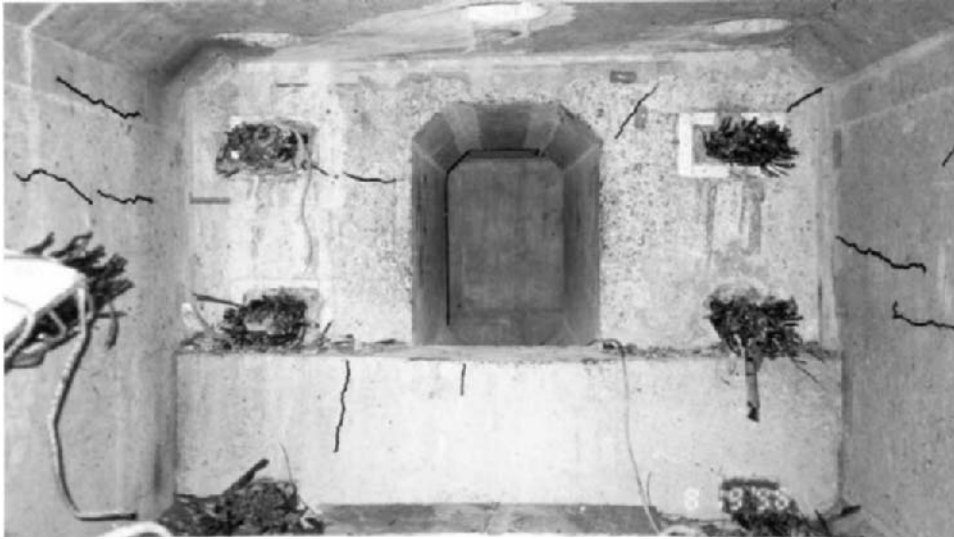
Figure 2.7 Cracking in a prestressed concrete box girder (cracks highlighted for clarity).
