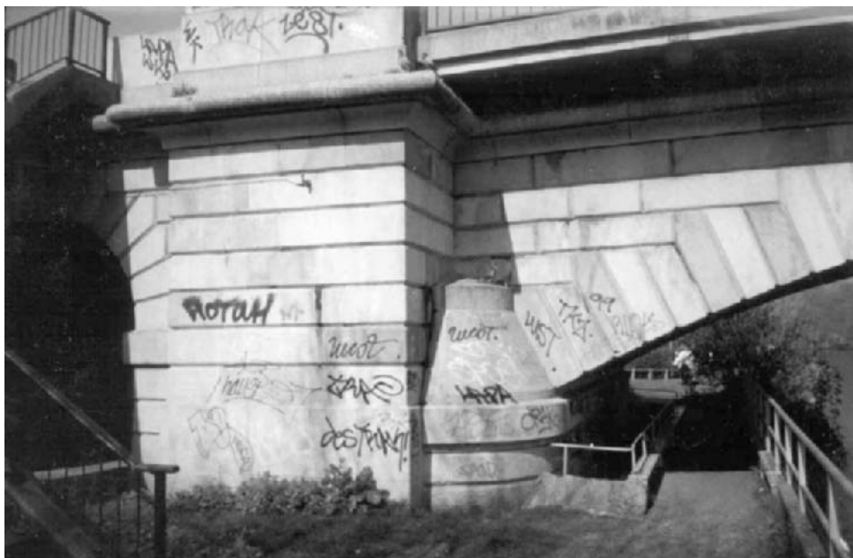
Figure 6.20 Graffiti on the abutment of an old arch bridge.
