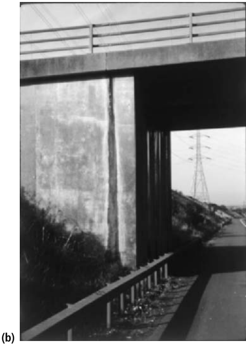
Figure 2.14 (a,b) Example of leaking joints.
