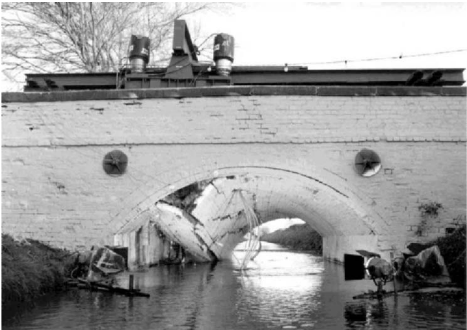
Figure 5.10 Collapse of the Torksey Bridge, UK (after Page, 1995) (photograph courtesy of TRL).
