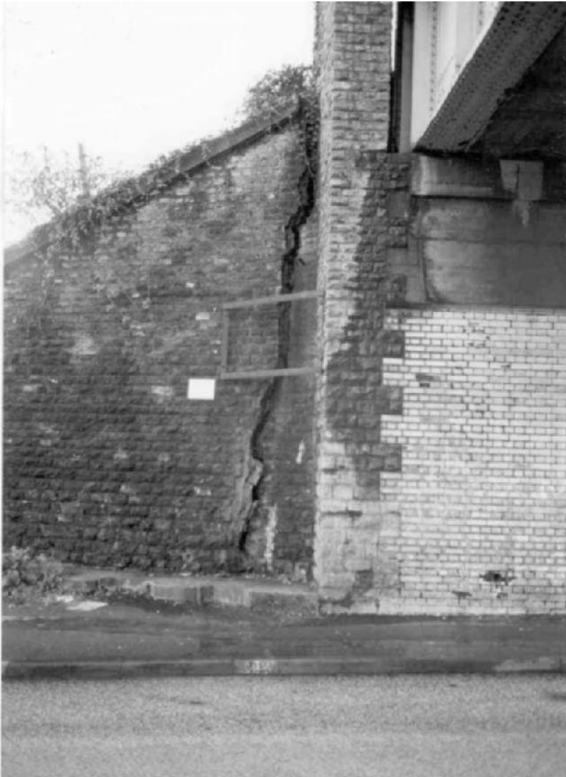
Figure 7.37 Cracking at abutment/wing wall intersection due to high soil pressures.
