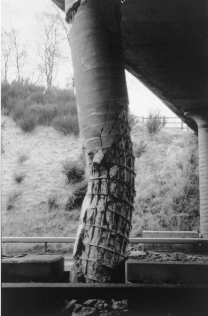
Figure 2.5(c) Example of bridge-bashing to a reinforced concrete pier.
