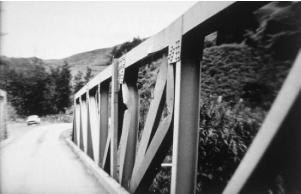
Figure 2.5(b) Example of bridge-bashing to a through-truss bridge.
