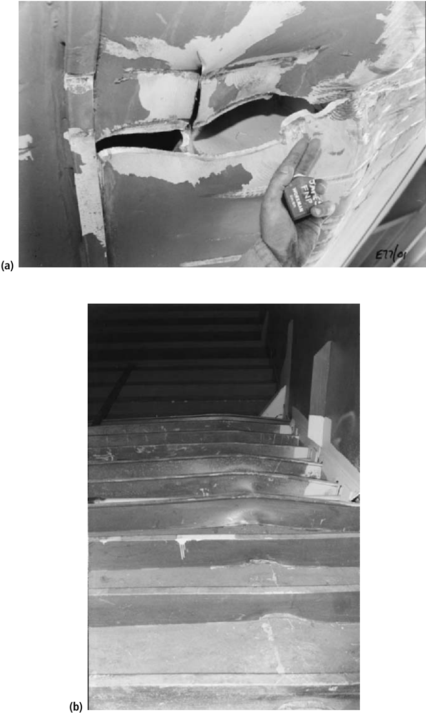
Figure 6.13 (a) Damage to bottom flange and (b) transverse stiffeners (courtesy Construction Repair ).
