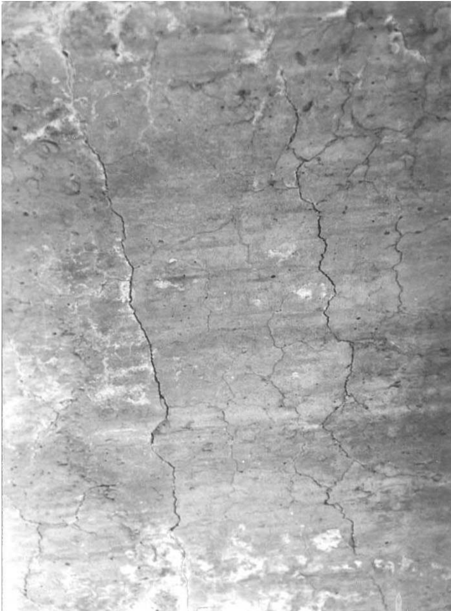
Figure 2.2 Cracking to the soffit of a slab.
