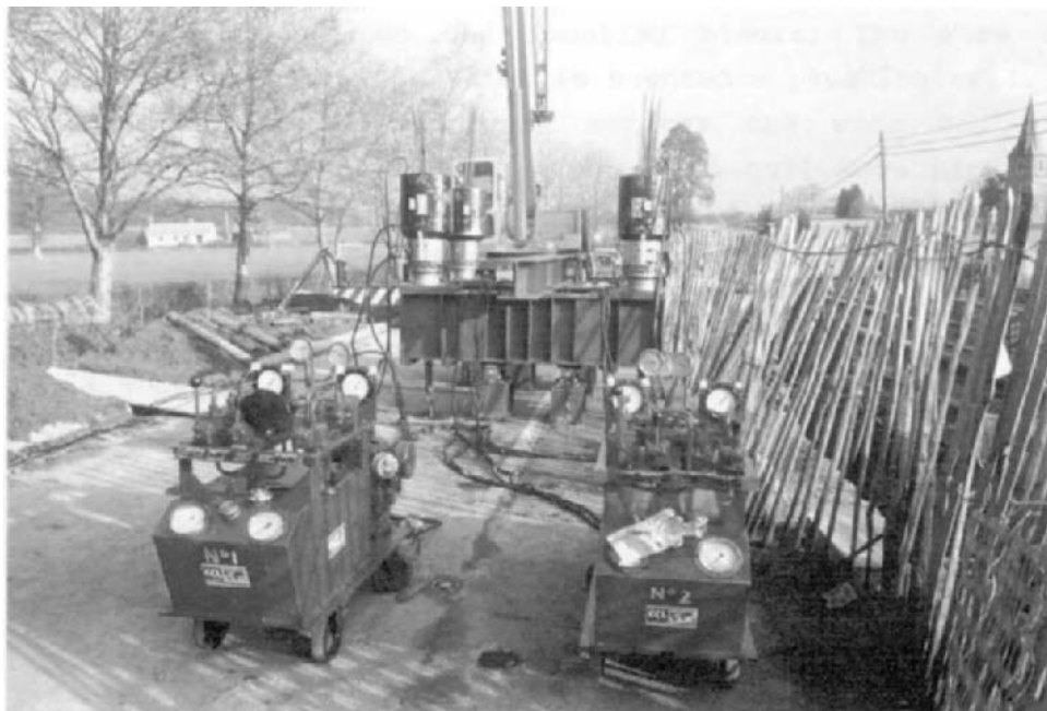
Figure 5.11 Typical loading frame for testing a shallow deck (courtesy of Ricketts, 1991).
