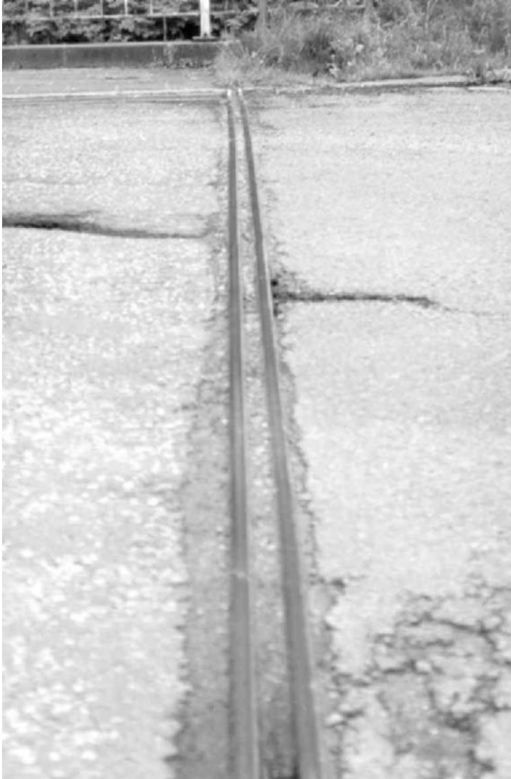
Figure 2.12 Example of tracking and cracking.
