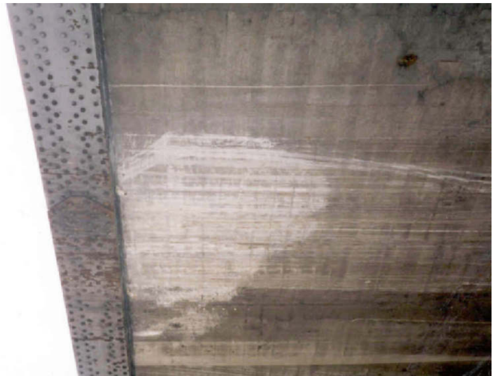
Figure 2.5(a) Example of bridge-bashing to the column of an overbridge.
