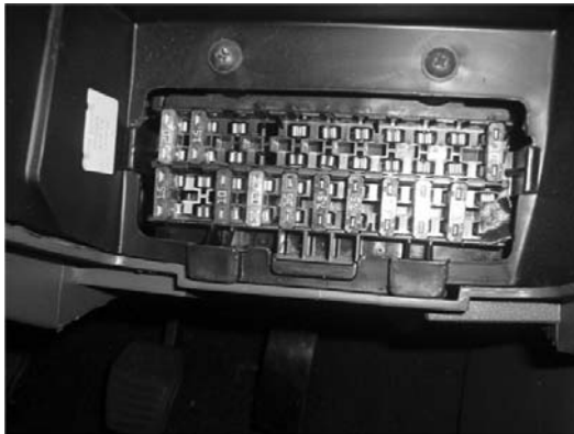
Figure 3.138 CJB, relays are behind the fuse box
