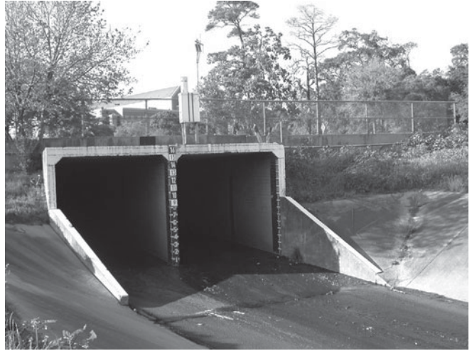
Drainage outlet with gage that monitors water flow.
