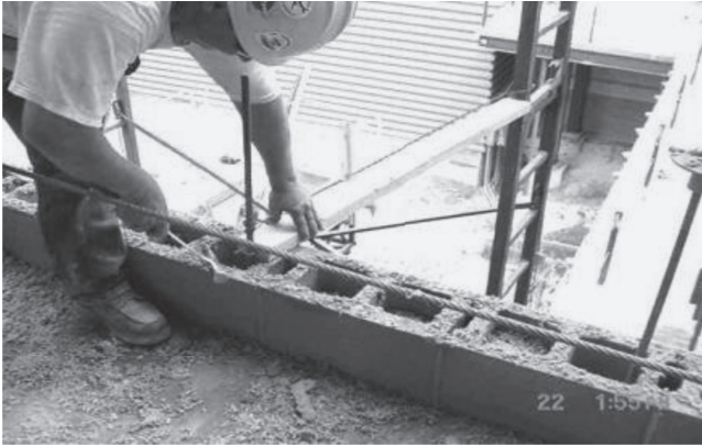
Protection often removed to work
