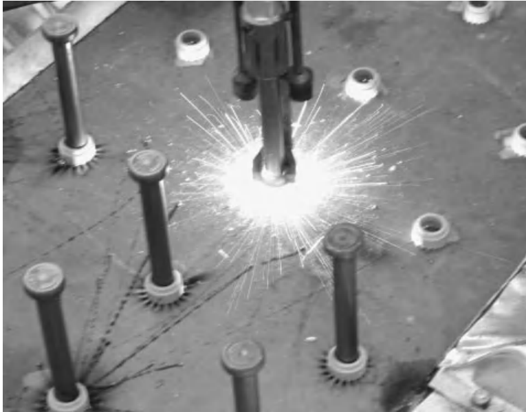
Figure 1.3-3 A steel shear stud being welded to the top flange of a steel beam.
