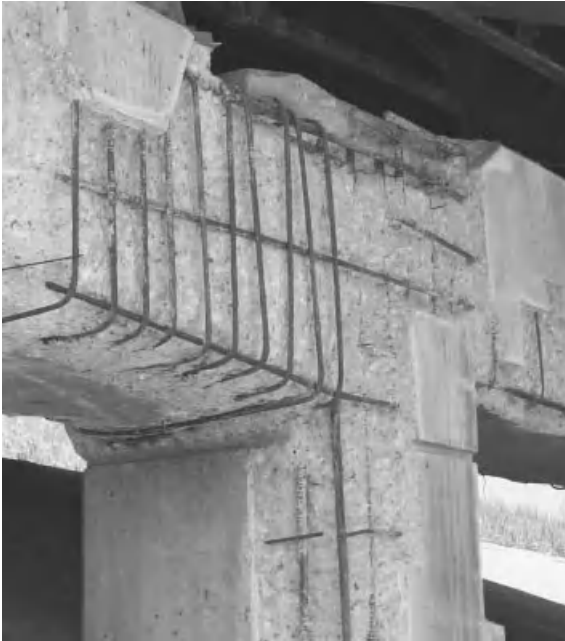
Figure 7.1-3 Reinforced concrete bridge pier with delaminated concrete marked and removed.
