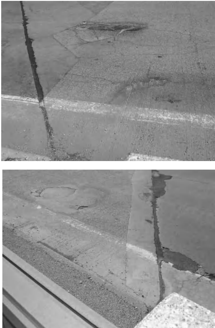
Figure 7.3-7 Concrete deck spalling (top) untreated and (bottom) patched.
