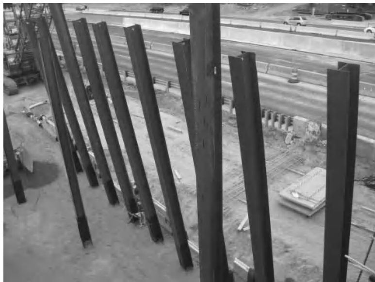
Figure 1.3-2 Steel piles placed as the foundation for an abutment to be constructed.
