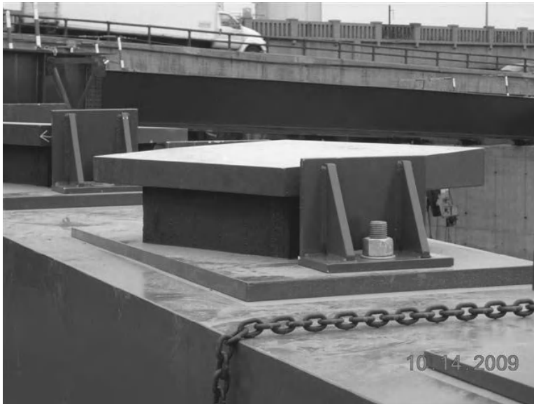
Figure 5.2-9 Elastomeric expansion bearing installed prior to erecting superstructure (Courtesy of the D. S. Brown Company, North Baltimore, OH).
