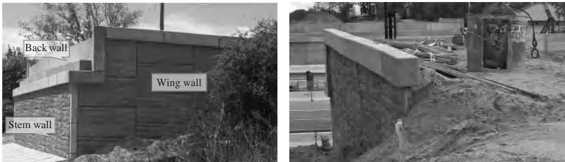
Figure 6.3-2 Full-height abutment with return wingwall with superstructure to be erected: (left) front view; (right) back view.
