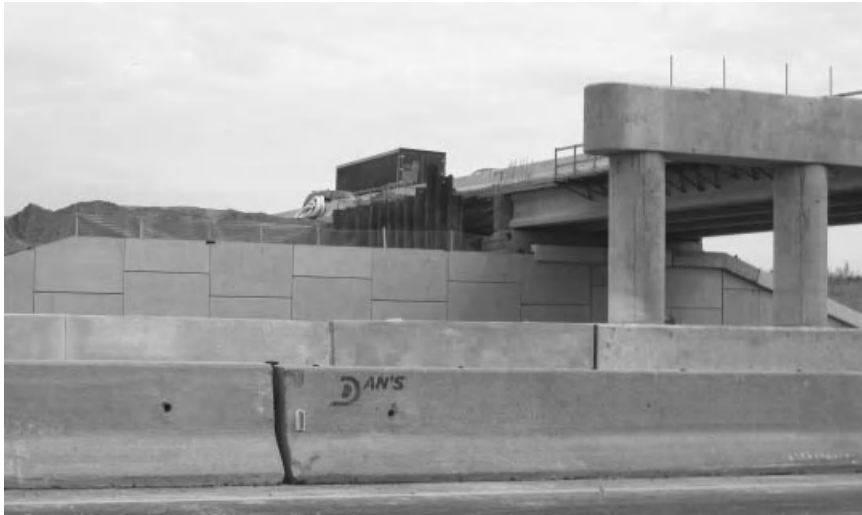
Figure 2.5-2 Replacing left half of the bridge while keeping the right half open.
