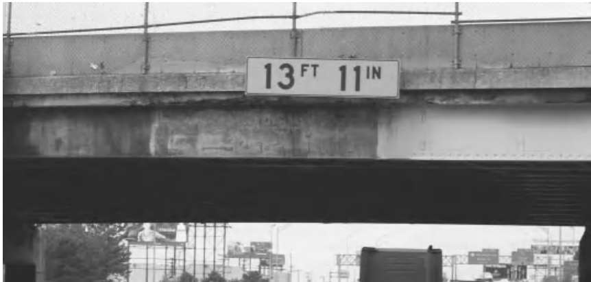
Figure 7.1-1 Steel bridge beam with corrosion and limited vertical clearance.
