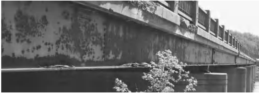
Figure 7.3-1 Significant paint damage and corrosion that may cause section loss.
