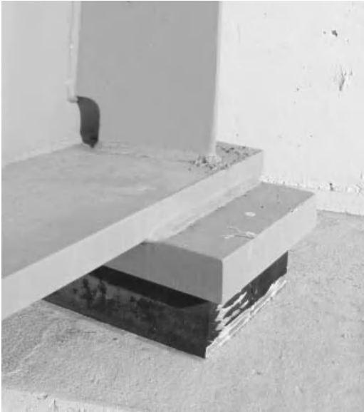
Figure 5.2-1 Elastomeric bearing supporting steel girder.
