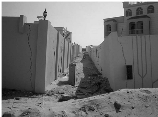
FIGURE 1.4 Cracks on the wall in Saudi Arabia.
