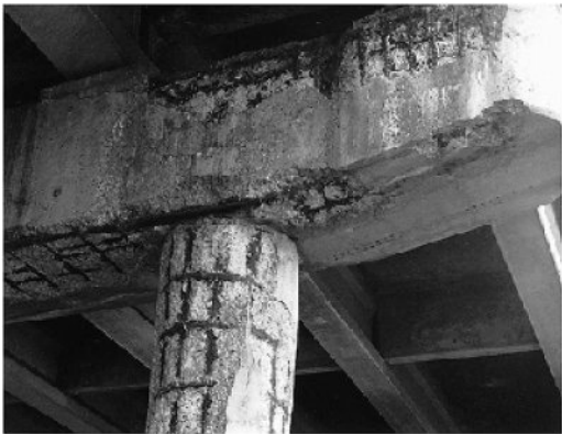
FIGURE 7.20 Corrosion on the main girder and columns for a bridge.
