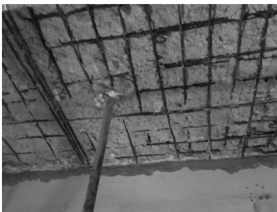
FIGURE 8.8 Corrosion of steel bars in slab.
