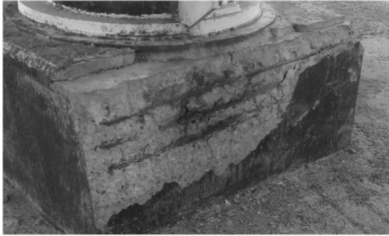
FIGURE 8.11 Corrosion in steel foundation under sphere tanks.
