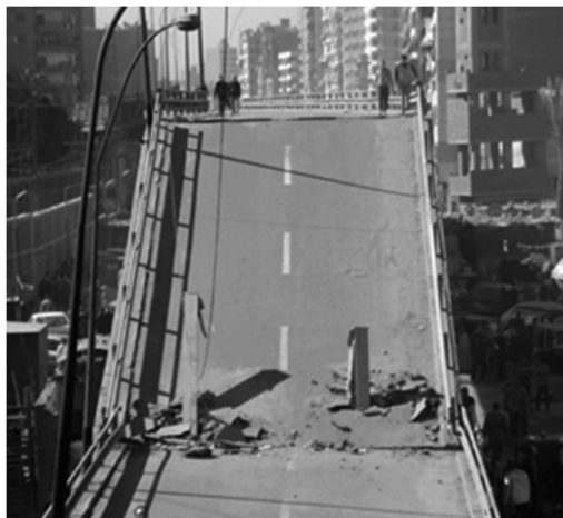
FIGURE 1.3 Bridge collapse in Egypt.
