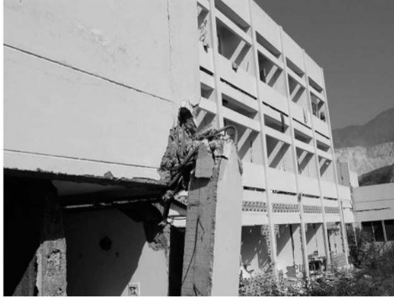
FIGURE 5.9 Large shear movement due to seismic load in Pakistan.
