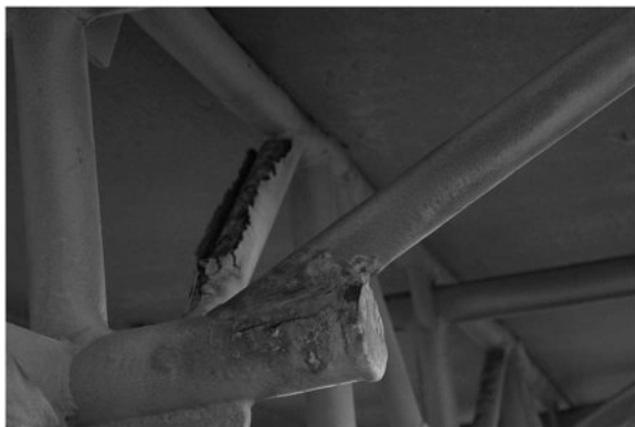
FIGURE 8.23 Corrosion of a truss member on a helideck.
