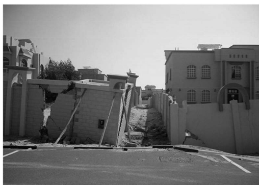
FIGURE 1.5 Wall inclination and cracks due to settlement.
