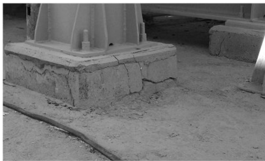
FIGURE 8.13 Corrosion in steel foundation under steel structure.
