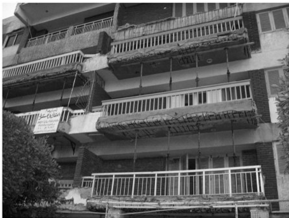
FIGURE 7.4 Corrosion of balconies.
