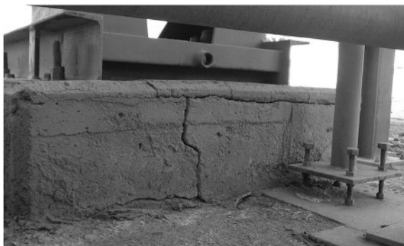
FIGURE 8.14 Corrosion in foundation under mechanical skid.
