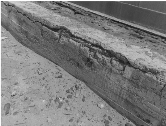
FIGURE 8.16 Ring beam failure
