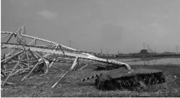
FIGURE 5.8 Collapse of Power Transmission Towers (Typhoon Higos, 2002).
