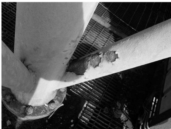
FIGURE 8.22 The corrosion on the tubular joint for the deck structure.
