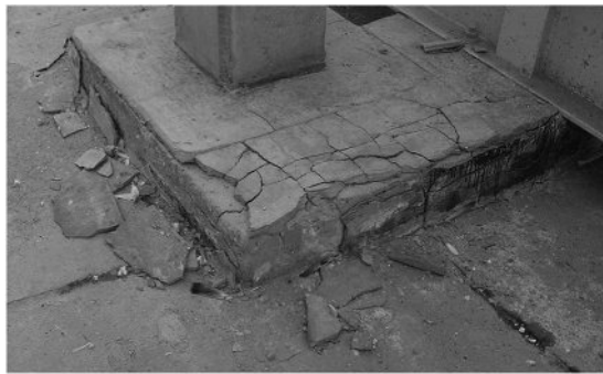
FIGURE 8.12 Corrosion in steel foundation under pipe support.
