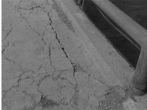
FIGURE 1.10 Harbor jetty failure.
