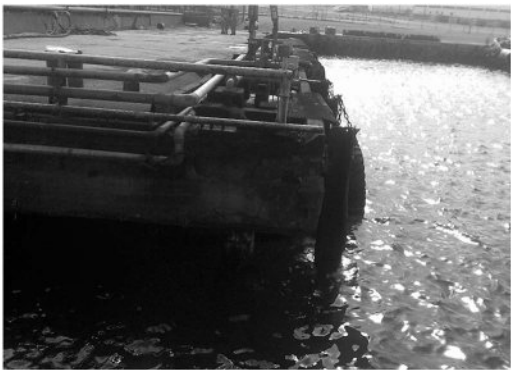
FIGURE 7.22 Corrosion of a jetty.
