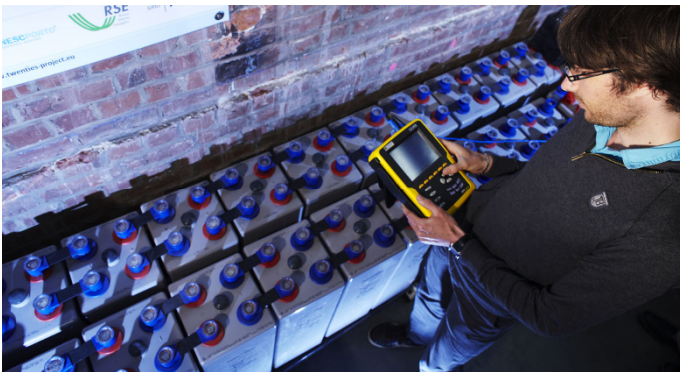
Figure 2.12. EnerSys lead batteries: 24 units, nominal voltage of 48 V, nominal current of 200 A, 10 kW power, 1,000 Ah capacity, discharge depth of 72.5% and number of complete cycles estimated at 1,335 (L2EP AMPT Lille)
