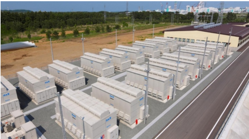
Figure 2.14. Seventeen groups of 2 MW of NaS batteries in Japan [KAW 10]
