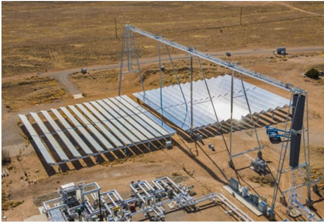
Figure 2.11. Utilization of molten salts as a heat-transferring fluid in a heliostatic solar power facility (source: Randy Montoya)
