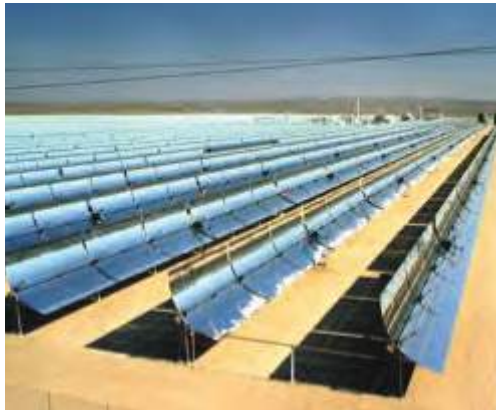
Parabolic Trough Concentrating Solar Collector at Kramer Junction, California Source: NREL 2012a
