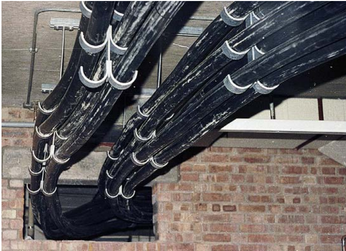
FIGURE 8.2 PVC/SWA/PVC sheathed cables being used as sub-main cables for distribution of power. Provision has been made for 12 240mm 2 four-core cables to be run, and in this view 11 have been fitted (William Steward & Co Ltd).
