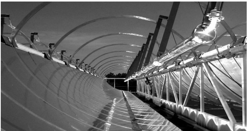
Figure 6.9 Passive parabolic concentrator installation. Courtesy of Solargenix.
