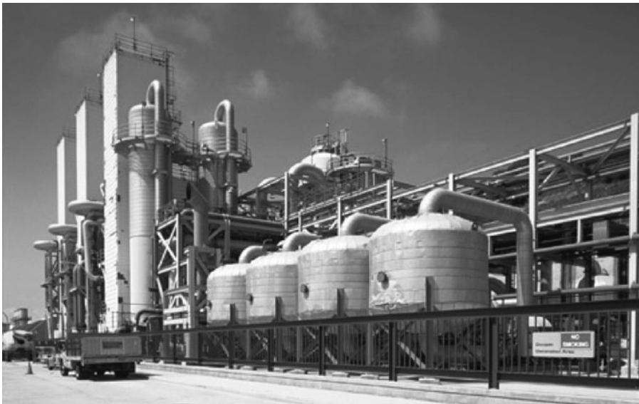
Figure 14.1 View of sedimentation tanks at the Hyperion Sewage Treatment Plant, Los Angeles, California. Courtesy of Hyperion.
