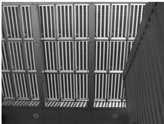
Figure 3.28 BIPV modules. Photo courtesy of Atlantis Energy Systems.
