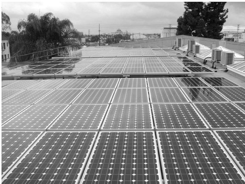
Figure 3.65 Roof-mounted solar power system, Arshag Dickranian School, Hollywood, California. Photo courtesy of Vector Delta Design Group, Inc.
