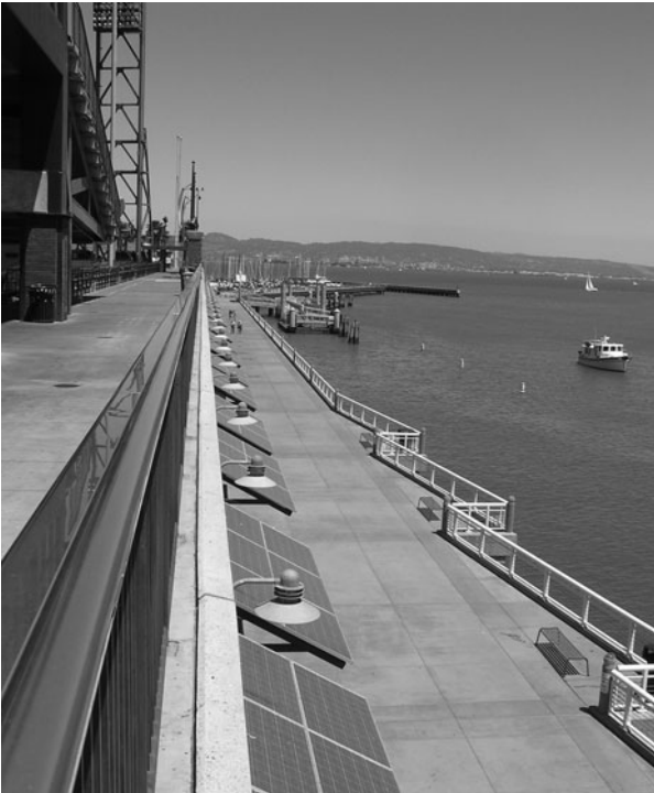
Figure B.13 Solar power window canopy. Photo courtesy of DWP Solar.
