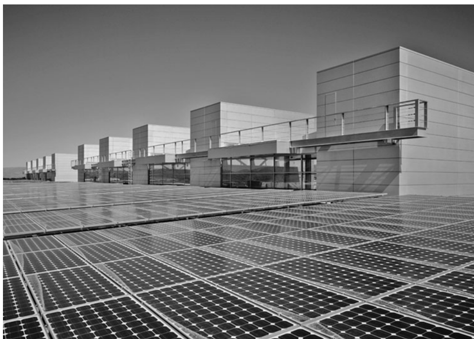
Figure 3.67 Water and Life Museum rooftop solar power system. Photo courtesy of Vector Delta Design Group, Inc.
