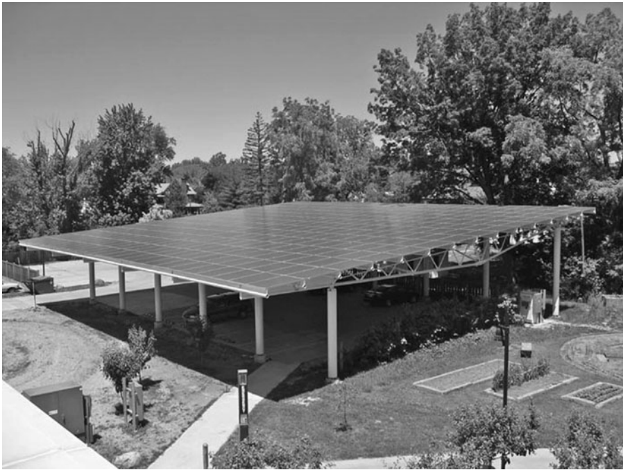
Figure B.4 Solar power parking canopy. Photo courtesy of DWP Solar.
