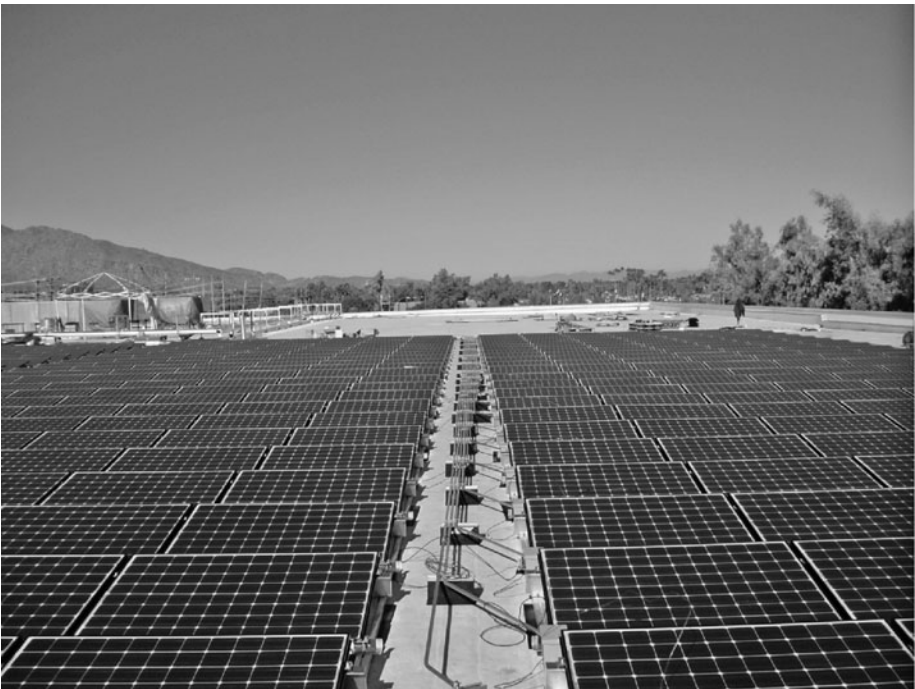
Figure B.17 Nonpenetrating-type roof-mount-solar power assembly. Photo courtesy of DWP Solar.
