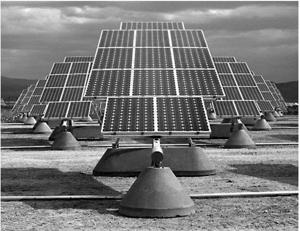
Figure 3.55 SunPower T20 single-axis solar power-tracking system. Photo courtesy of SunPower.
