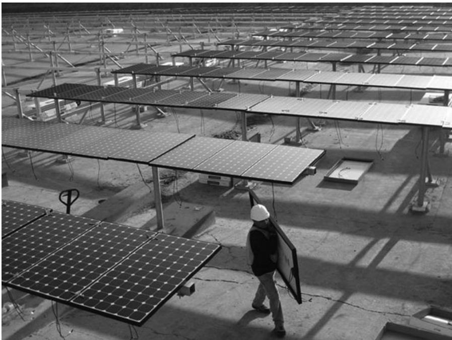
Figure B.11 Ground-mount solar power. Photo courtesy of A&M Energy Solutions.
