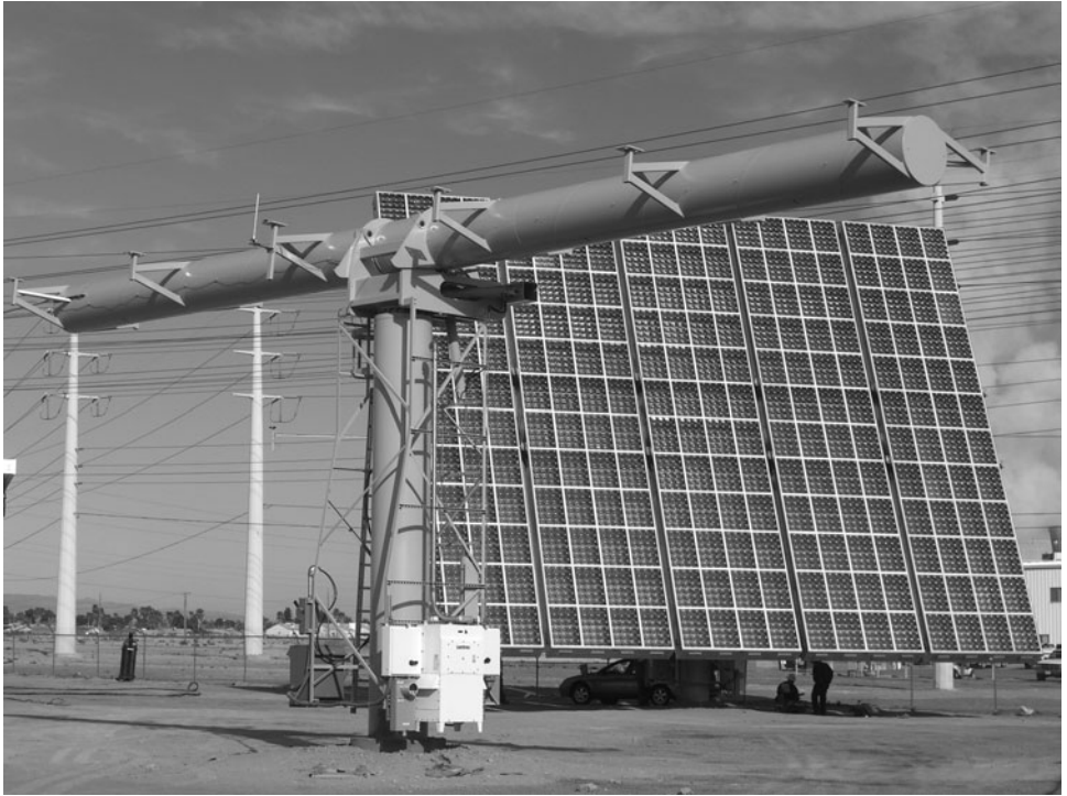
Figure 3.22 Amonix MegaConcentrator hydraulic arm assembly. Photo courtesy of Amonix.
