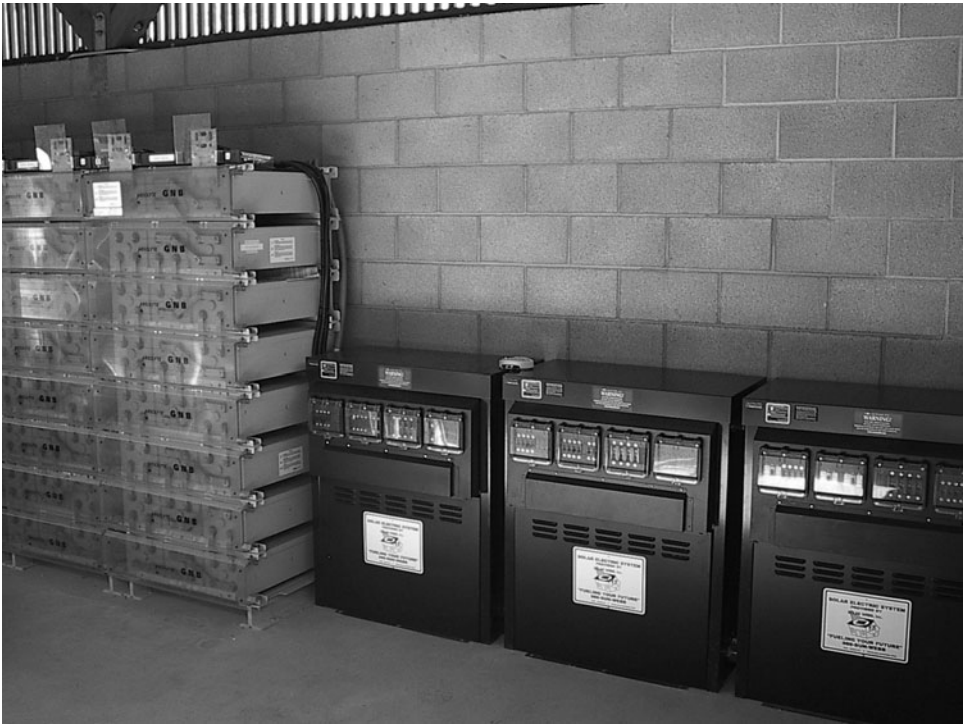
Figure 3.43 Deep-cycle battery packs. Photo courtesy of Solar Integrated Technologies.
