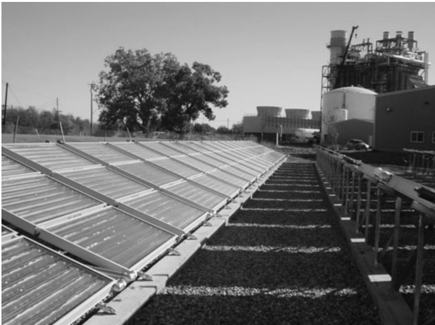
Figure 6.7 An industrial solar water-heating panel installation.
