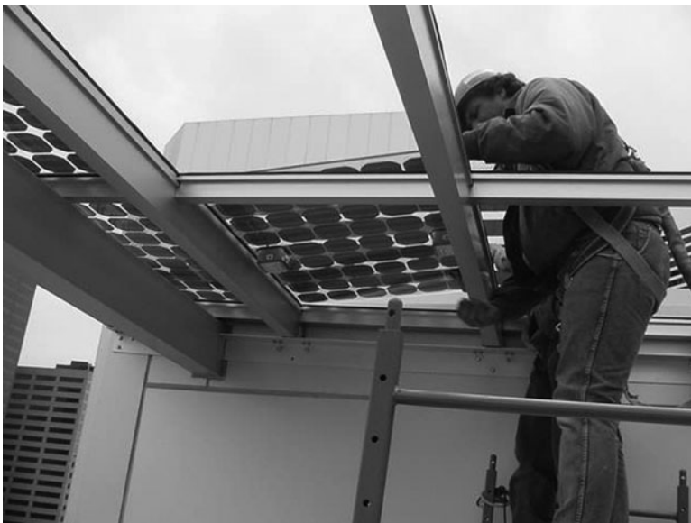
Figure B.5 Building-integrated solar power. Photo courtesy of Atlantis Energy.
