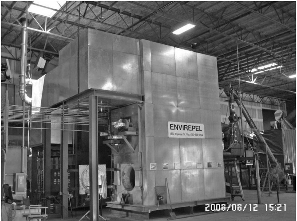
Figure 12.13 A biofuel-production plant. Courtesy of MARTIFER.
