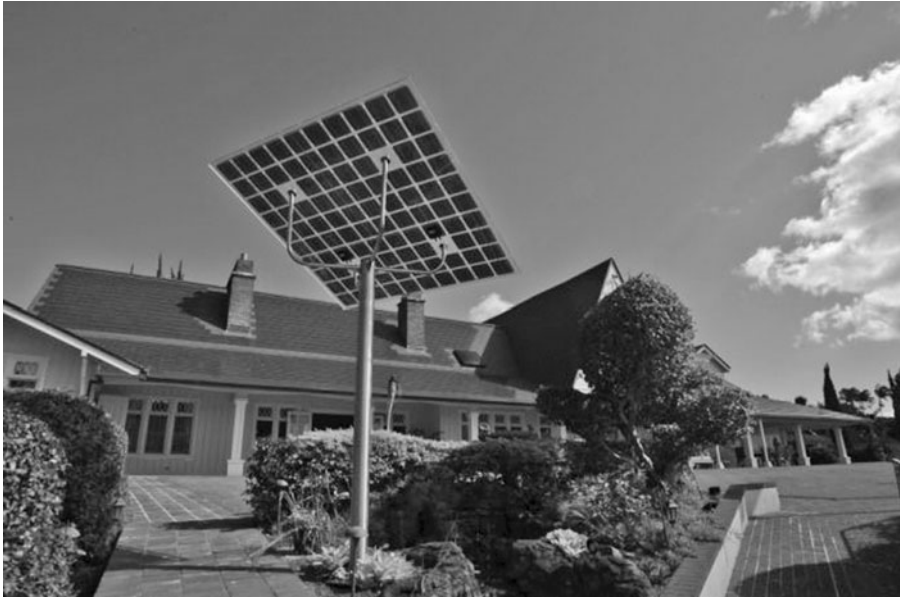
Figure B.8 Building-integrated solar power stand. Photo courtesy of DWP Solar.
