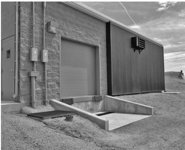
Figure 6.4 Industrial passive solar water-heating system.
