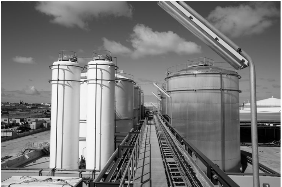
Figure 12.12 Photograph of Envirepel biomass energy plant.
