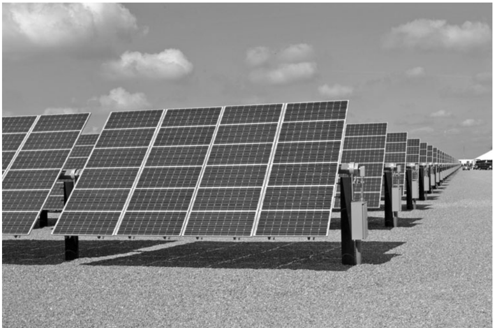
Figure 3.71 A large-scale single-axis solar farming system, Semitropic Water District, Wasco, California. Photo courtesy of SolarWorld.
