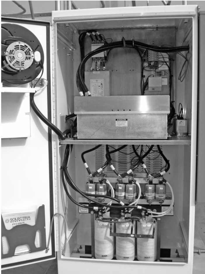
Figure 3.13 Internal view of inverter electronics. Photo courtesy of Solectria Renewables.
