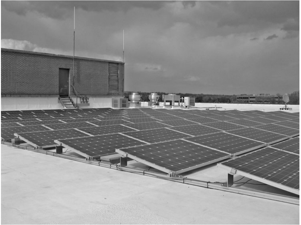
Figure 3.68 Nonpenetrating roof-mounted solar power installation with adjustable tilt support platform. Photo courtesy of DPW Solar.
