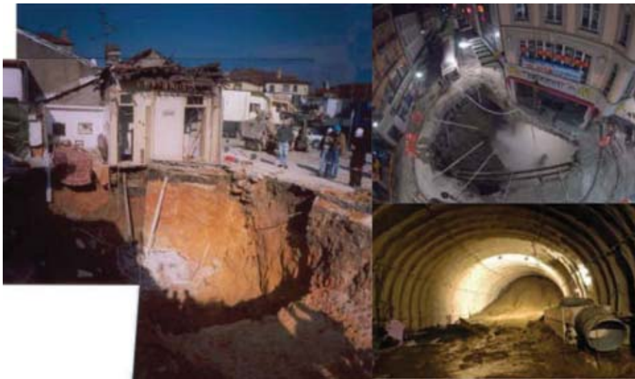
Figure 6.1 Some pictures of collapse consequences.
