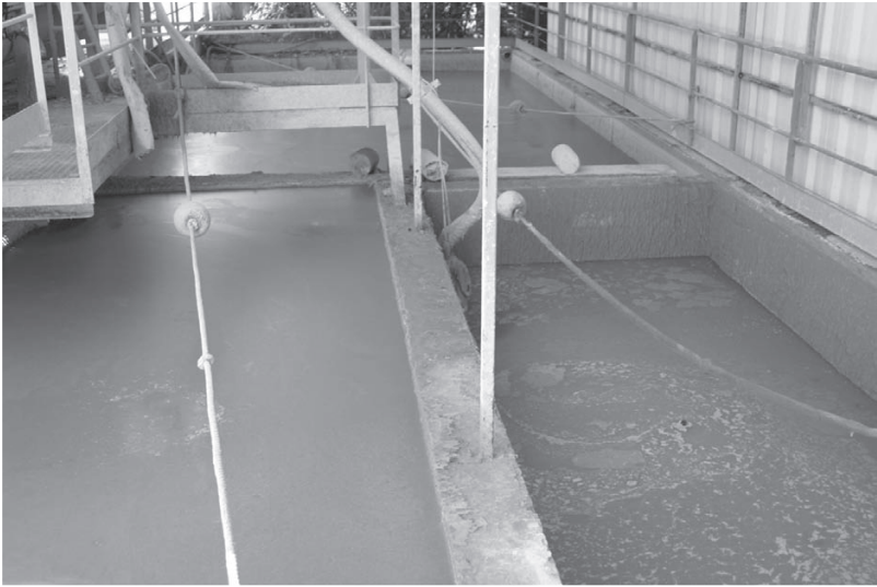
Figure 17.15 Sedimentation basins; Italcimenti plant at Biarritz.
