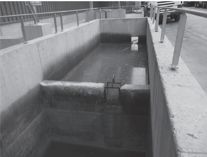
Figure 17.6 Decantation of the charged water; Cemex plant at Ivry.
