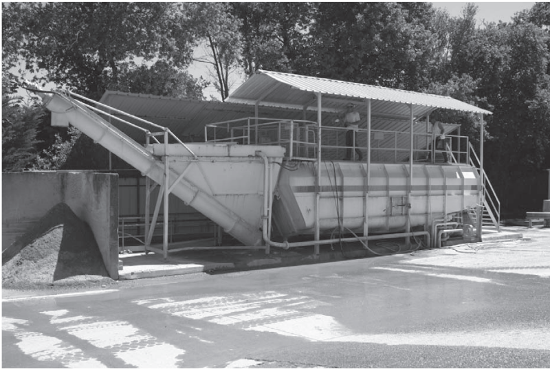
Figure 17.12 The treatment unit; Italcimenti plant at Biarritz.
