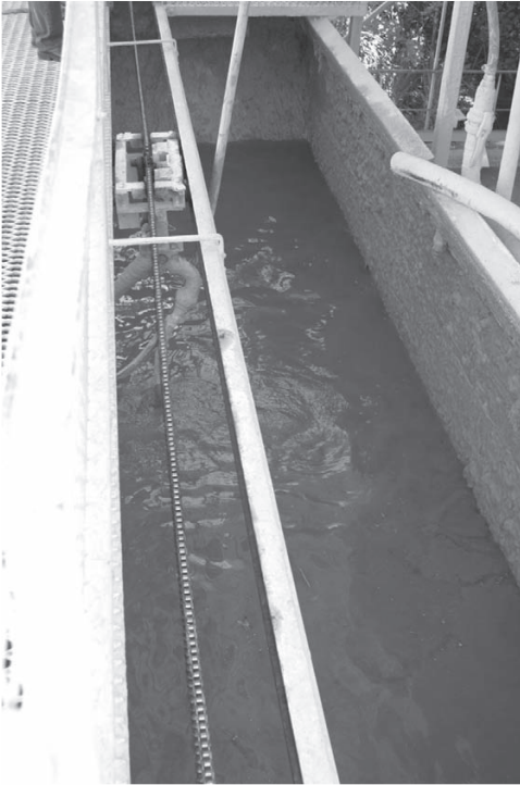
Figure 17.14 Charged water basin; Italcementi plant at Biarritz.
