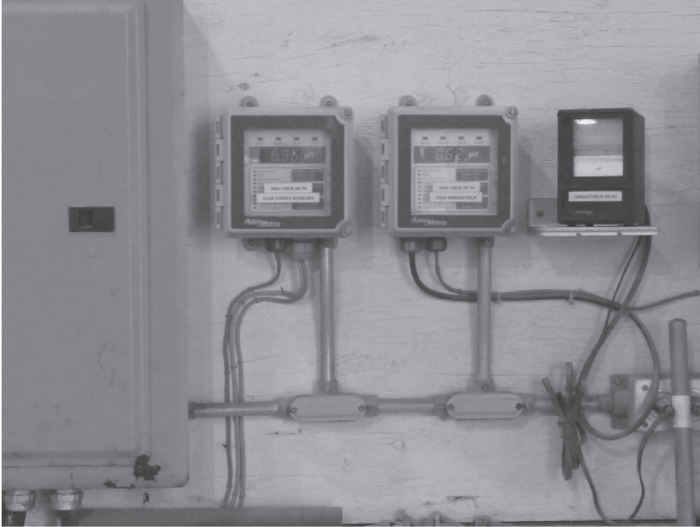
Figure 17.20 pH control of the treated water; Demix Béton plant.
