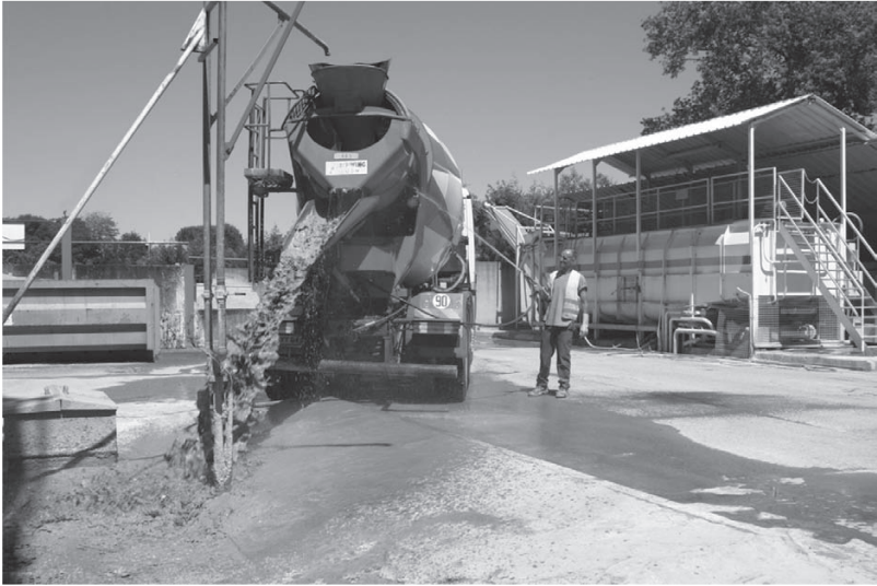
Figure 17.9 Cleaning a truck in the decantation pit; Italcimenti plant at Biarritz.
