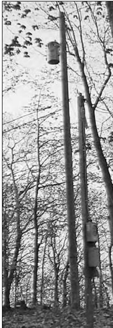
Figure 2-3: Temporary service panels usually look something like this.
