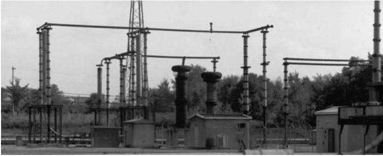
FIGURE 6.10 800-kV dc terminals of a converter station.
