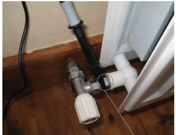
Unpainted metal work
