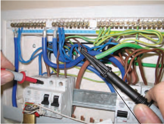
Connections for 2-lead instrument Disconnected earthing conductor
