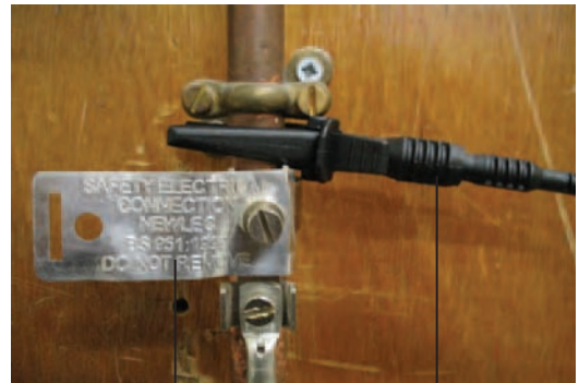
Banded metalwork Other end of test lead
