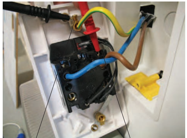
Test instrument probe at incoming CPC terminal of switch
