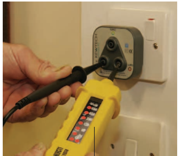
No voltage lights lit
