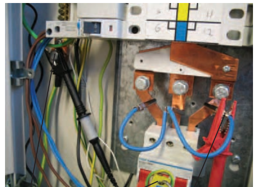
Earth Locked off and isolated All phases joined together
