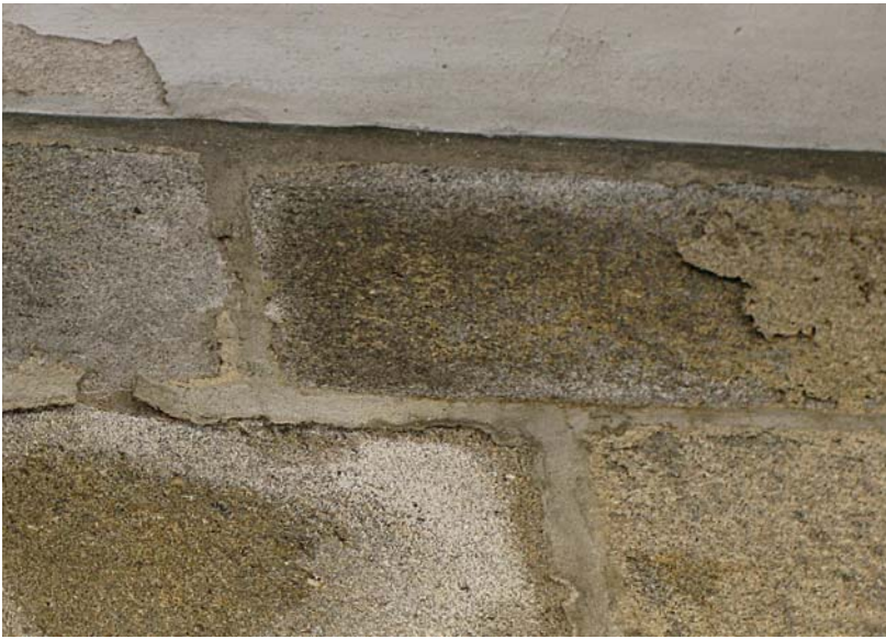
Figure 8. Black crusts on granite stones (a) and efflorescences and planar detachments on a granite wall.
