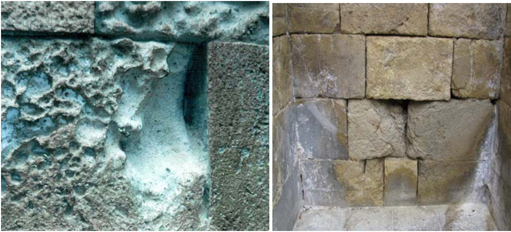
Figure 1. Examples of stone decay features: carbonate crusts on granite (a) and erosion of surface in stones made from volcanic rocks (b), granite (c) and limestone (d).
