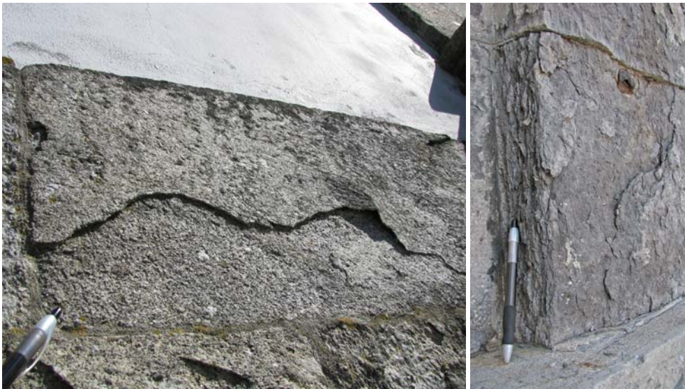
Figure 3. Planar detachments in granite (a) and sedimentary stones (b, note the clear influence of the rock structure).
