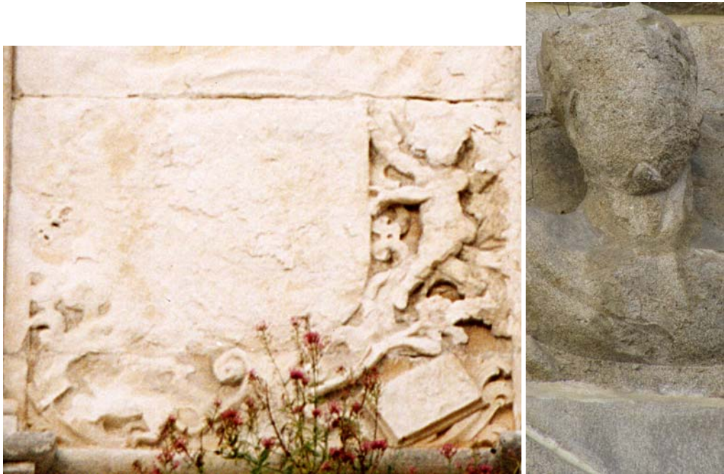
Figure 2. Erosion of surface causing damage to artistic stone works in limestone (a) and granite (b) stones.
