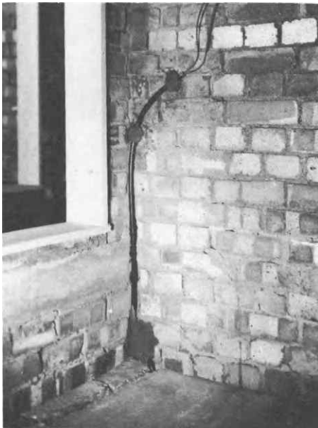
Fig. 8.18. Flexible non-metallic conduit drop to switch point run in wall angle to avoid wall chasing. Conduit is held in position with cement
