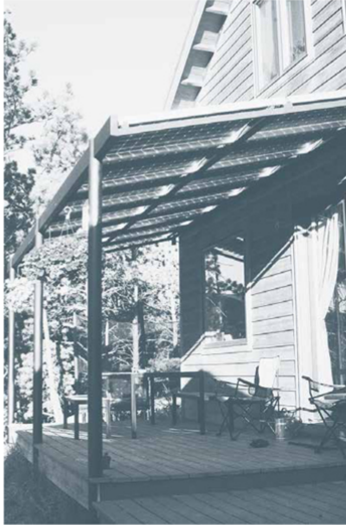
Figure 3.10. PV Awning. Solar awnings, like the one shown here, provide shade for windows and walls, eliminating the need for conventional awnings. Like other forms of building-integrated PVs, they perform more than one function. Awnings shade windows and walls and thus cool buildings in the summer and produce electricity year round. Credit: Lighthouse Solar, Boulder, CO.
