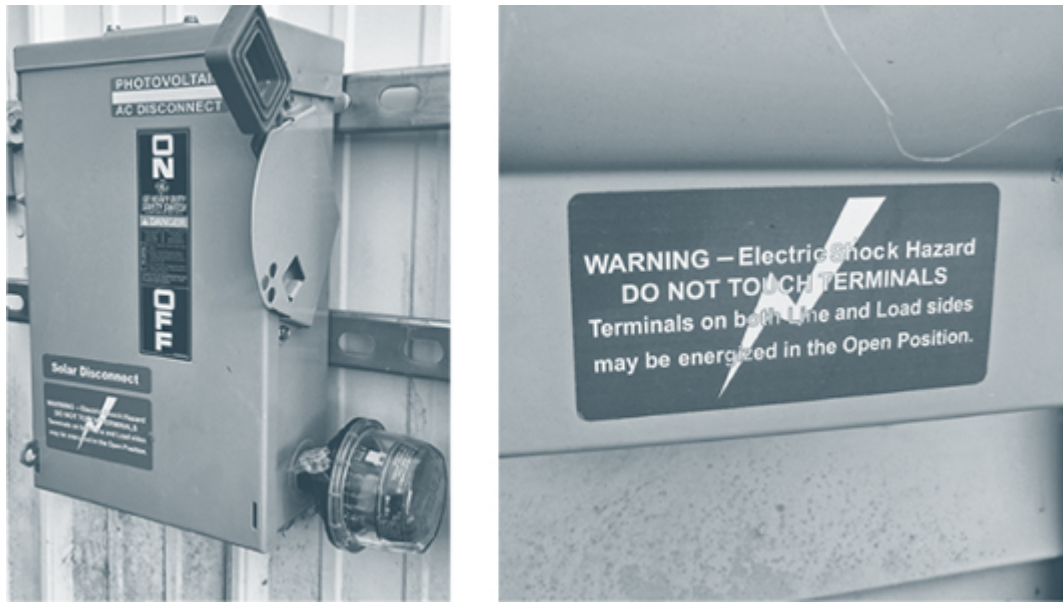
Figure 5.9. Label on Utility Disconnect. Utility disconnects like the one shown here must, according to the National Electric Code, be properly labeled to warn electricians that even though the switch is open, the terminals can be live (right panel). Notice the surge protector on the side of the disconnect (left panel) and the hole in the switch handle through which the utility inserts its lock should they need to lock a system out of the utility network for repair. Utilities typically require installers to mount the AC disconnect close to the utility meter. Credit: Dan Chiras.
