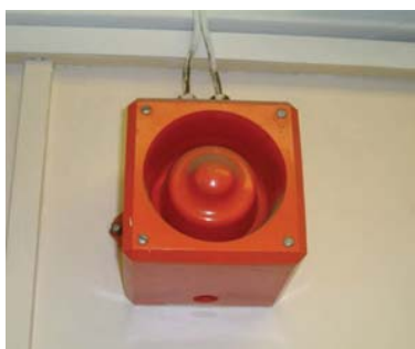
Figure 9.81 Audible fire alarm
