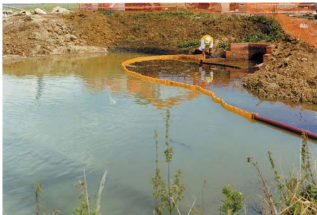
Figure 13.9 A boom designed to limit contamination
