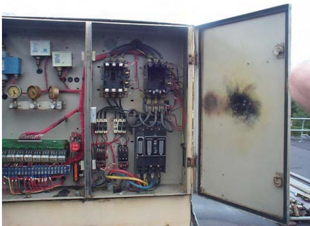
Figure 12.20 Damage to electrical distribution cupboard
