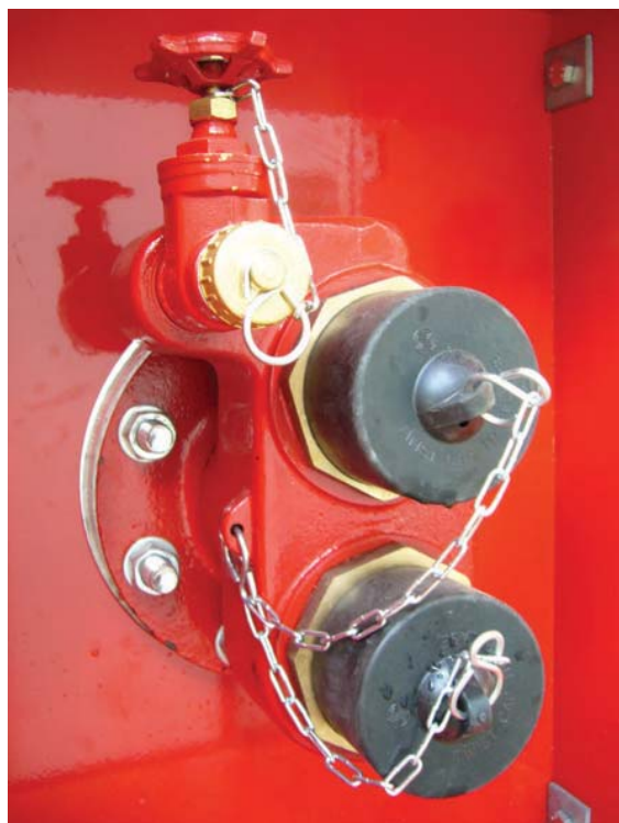
Figure 9.88 Dry riser outlet
