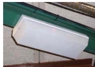
Figure 9.55 Non-maintained satellite emergency light
