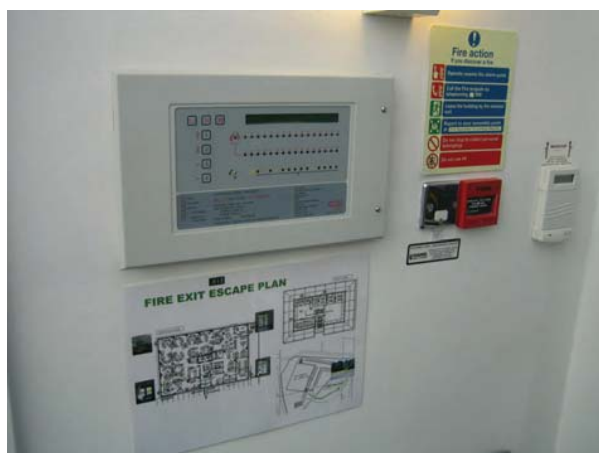
Figure 9.79 Typical fire alarm panel
