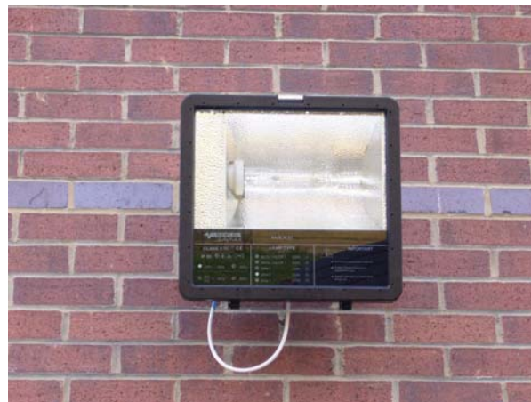
Figure 8.9 Typical security lighting
