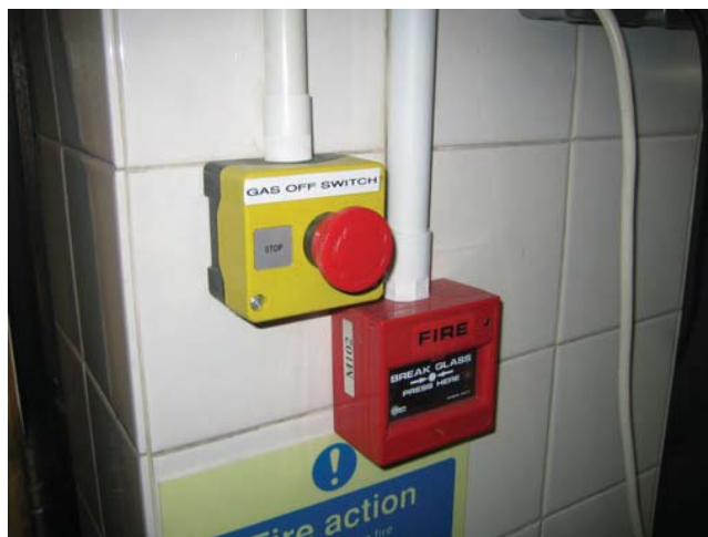
Figure 3.10 Isolation switch for gas-fired kitchen equipment
