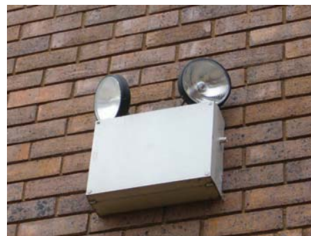
Figure 9.51 Emergency lighting unit
