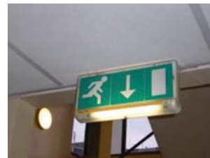
Figure 9.53 Maintained emergency exit box
