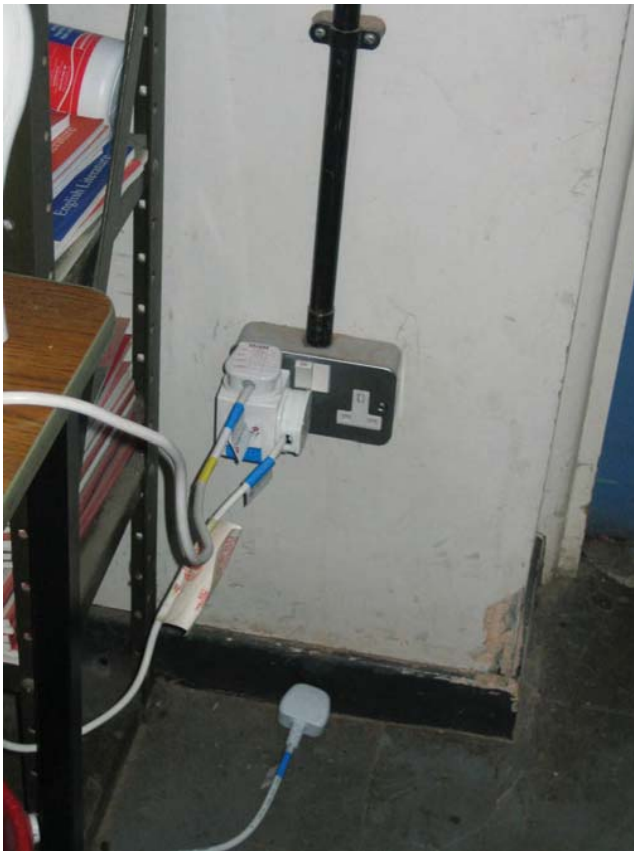
Figure 11.6 Misuse of electrical adaptors
