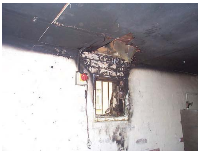
Figure 12.19 Damage to Vent Axia
