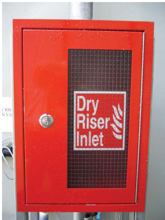
Figure 9.87 Dry riser inlet
