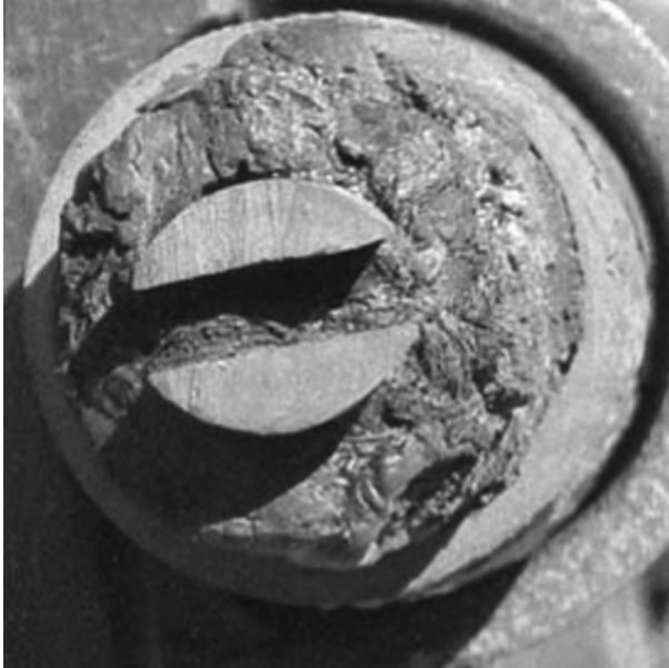
FIGURE 1.1 Early Edison cable. Photos courtesy of Robert Lobenstein/IEEE Power & Energy.
