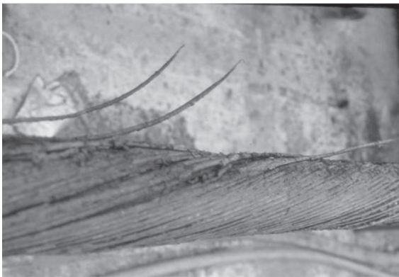
FIGURE 23.3 Steel armor wires corroded by AC current.
