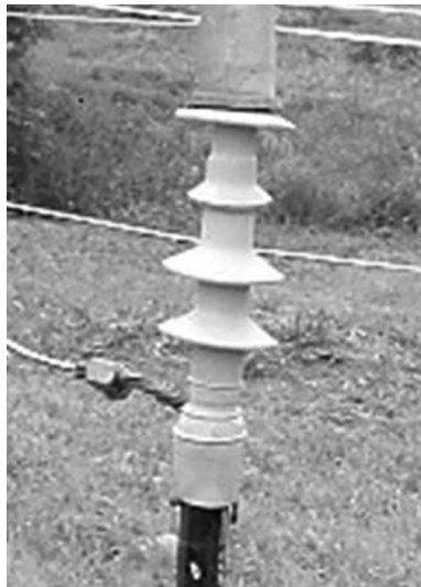
FIGURE 13.6 Cold shrink termination with skirts.
