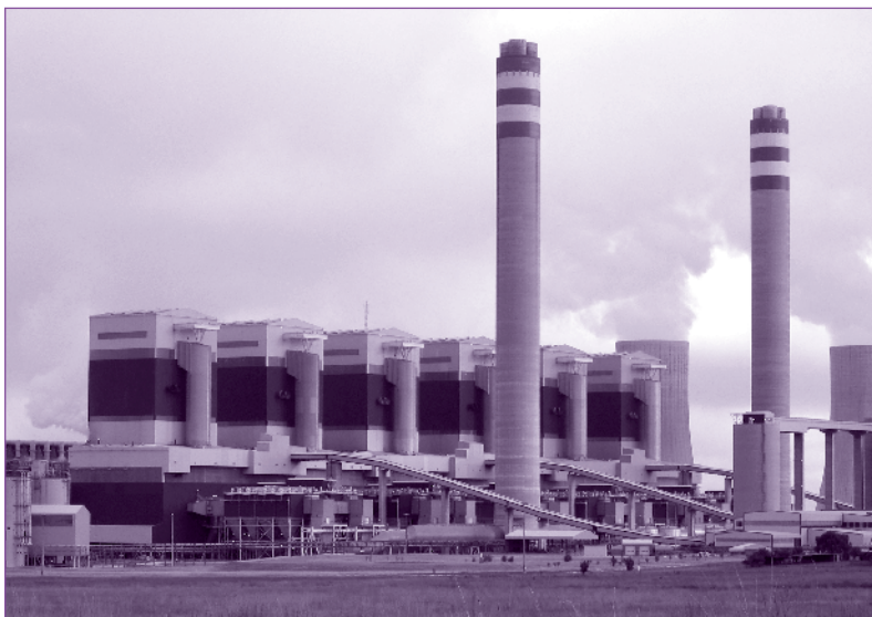
Figure 23 • Majuba power station
