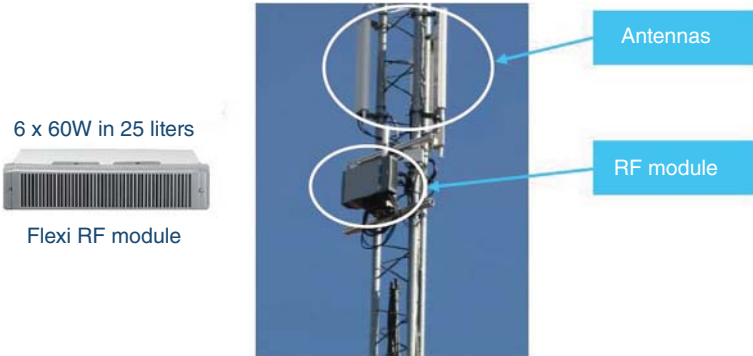
Figure 14.8 Compact Nokia RF module site solutions [9].
