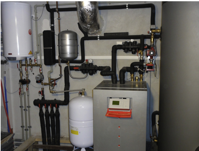
FIGURE 7.4 Solar combi heating system (indoor part, i.e., excluding solar collectors) cooperation with a ground heat pump.
