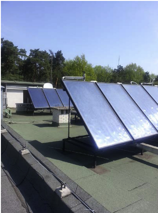
FIGURE 7.2 Solar collectors installed on a hospital roof in Konstancin, Poland.
