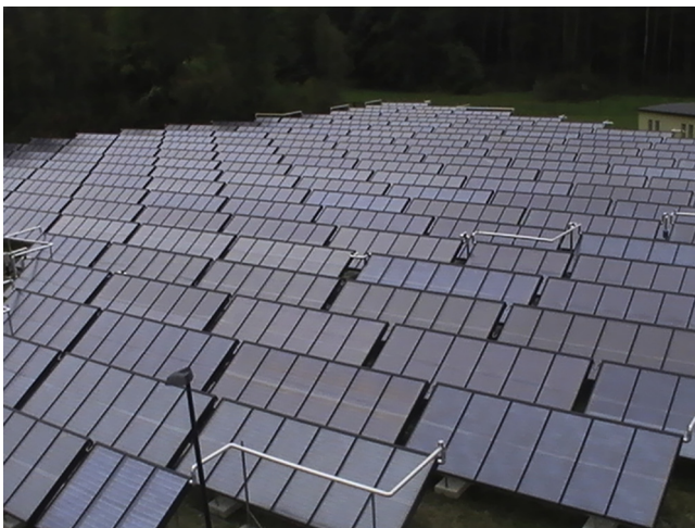
FIGURE 7.3 Solar collectors in a centralized solar heating plant in Graz, Austria.
