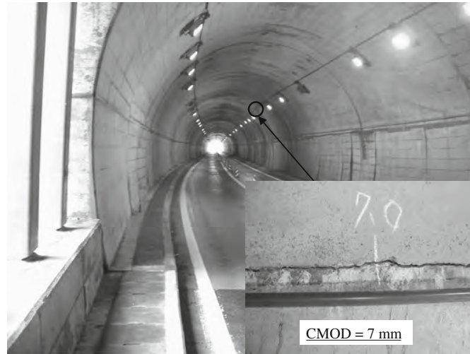
PHOTO 1.1 A highway tunnel with a large longitudinal crack in the right arch area.
