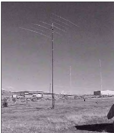
Fig 18 —Installation of surplus AB-577 tower with triband at 45 feet at K7NV. (Photo by Kurt Andress, K7NV)
