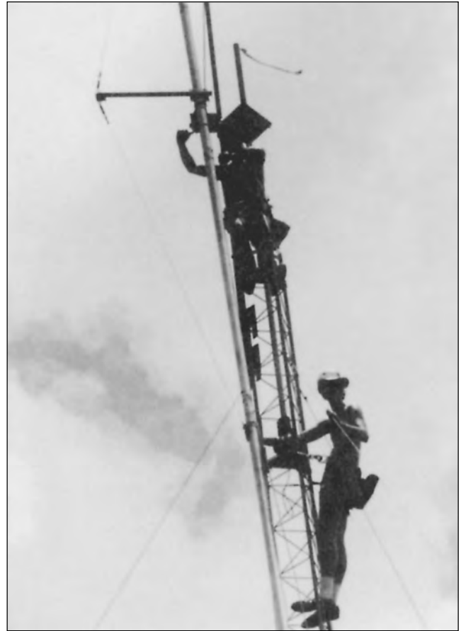
Fig 39—Working at the 70-foot level. A gin pole makes pulling up and mounting the boom to the boom plate a safe and easy procedure.
