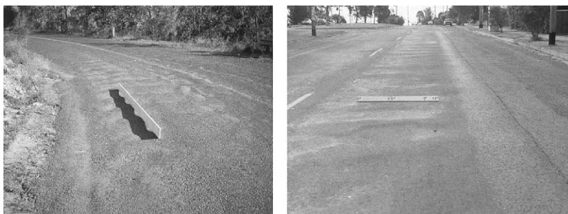
FIGURE 19.4 Corrugations in flexible pavements (Source: Austroads, 1987).
