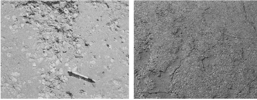
FIGURE 19.20 Raveling in flexible pavements (Source: Austroads, 1987).
