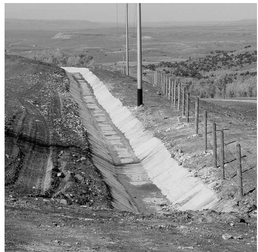
FIGURE 13.6 Concrete linked ditch.
