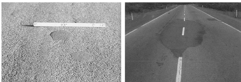
FIGURE 19.23 Patches in flexible pavements (Source: Austroads, 1987).
