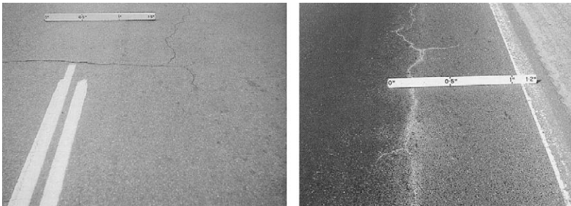
FIGURE 19.15 Meandering cracks in flexible pavements (Source: Austroads, 1987).
