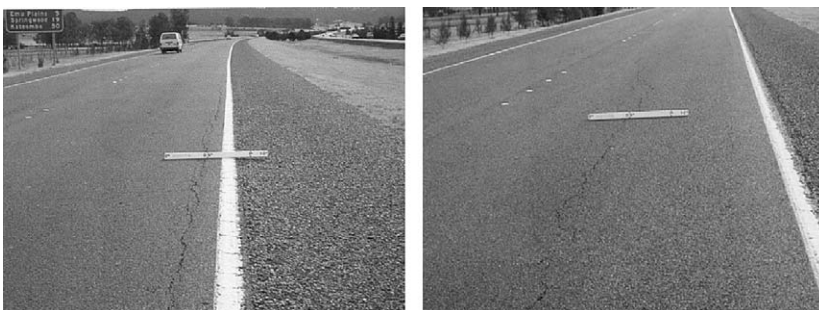
FIGURE 19.10 Longitudinal cracks in flexible pavements (Source: Austroads, 1987).
