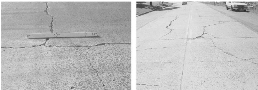
FIGURE 19.32 Block cracks in rigid pavements (Source: Austroads, 1987).
