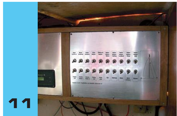
▲ The first test went well. To finish, all the loose cables around the cabinet need to be tidied up.
