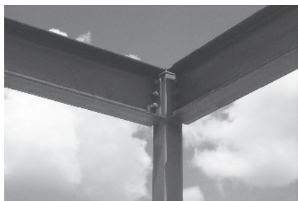
Pin-connected steel members.
