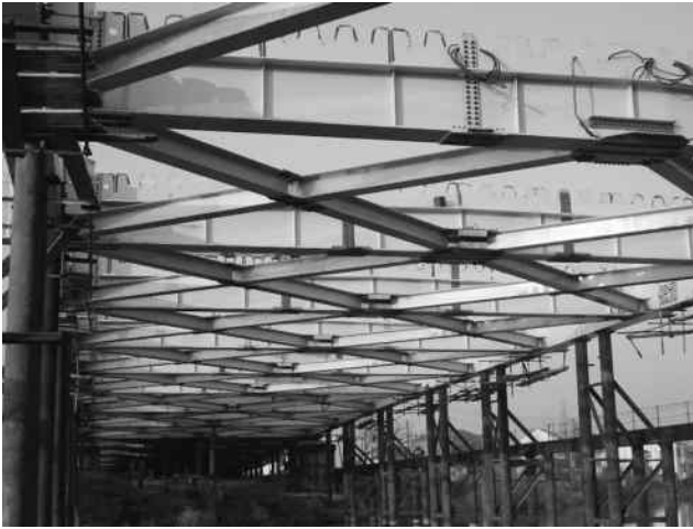
Figure 10.36 Rigid connections of Shang Xin Bridge.
