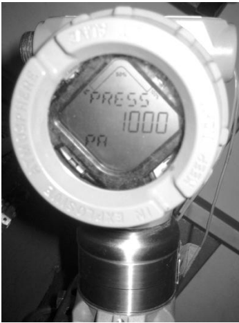
Figure 15.23: Differential pressure transmitter operating on a 4 - 20 mA Current Loop. Display shows pressure in Pa.
