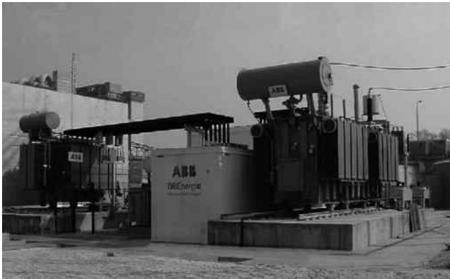
Fig. 13.8b: 15-MW standard railway supply converter (ABB Switzerland AG)
