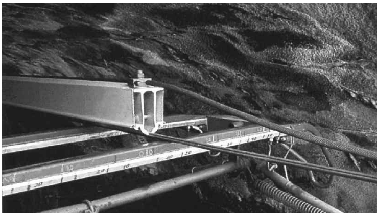
Fig. 13.20: Overhead conductor rail (left), transition to standard catenary, pantograph head with earthed horns (AVG Karlsruhe)
