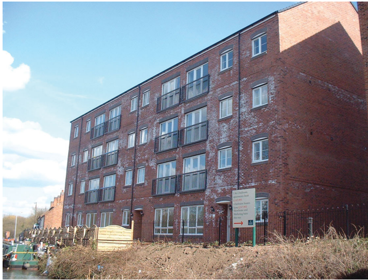
FIGURE 34.4 Severe Efflorescence on New Brickwork
