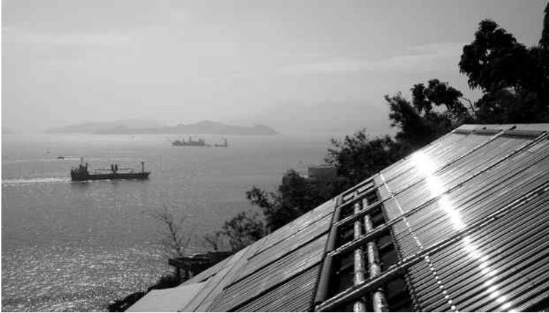
Figure 5.1 A domestic solar thermal system installed on the roof of a house in Hong Kong (Photo courtesy: Mr. Jackson FUNG)
