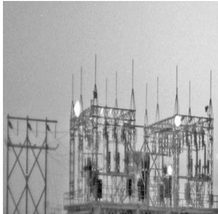
FIGURE 12.17 Switchyard protected by masts
