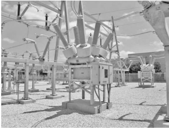
FIGURE 7.8 SF 6 gas circuit breakers
