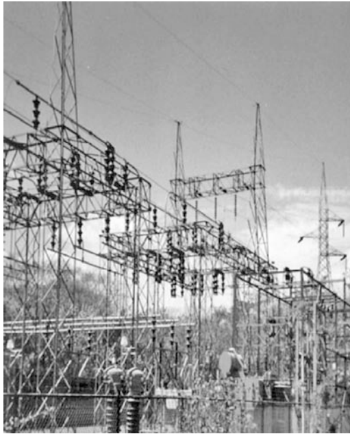
FIGURE 12.16 Switchyard protected by overhead shield wires
