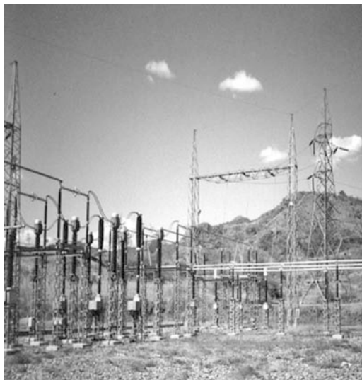
FIGURE 12.14 Switchyard using rigid bus-work
