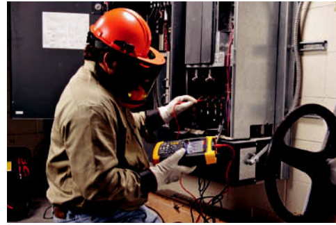
Figure 10-30 Taking measurements on a VFD.
