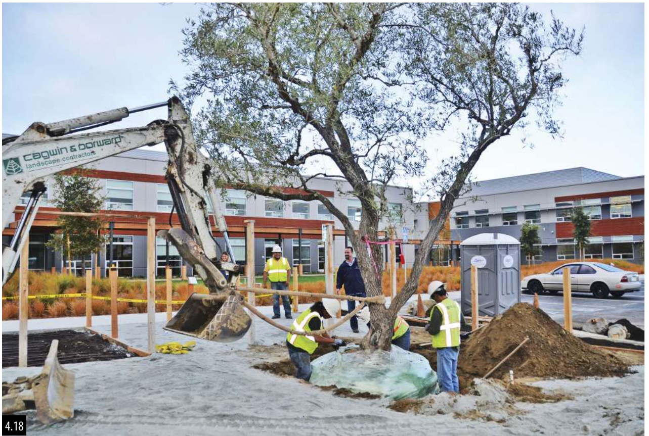
Figure 4.17 At VF Outdoors in Alameda, California, a heritage California Mission olive tree being placed in the field before the remaining edible garden is constructed. Scheduling is an important part of the process.
