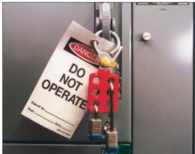
FIGURE 3-4 Multiple locking device shows that the equipment can be locked out by several different people.
