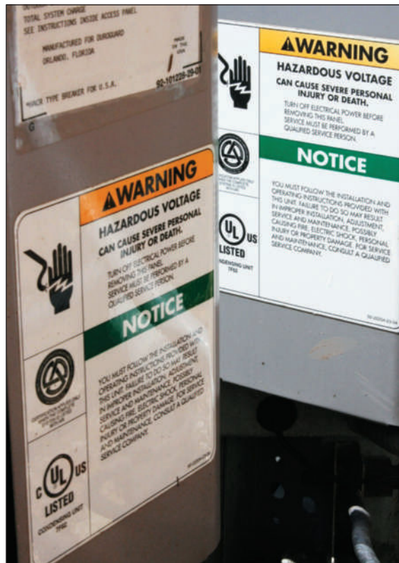
FIGURE 10-20 These HVAC units show a typical placement of the UL logo.
