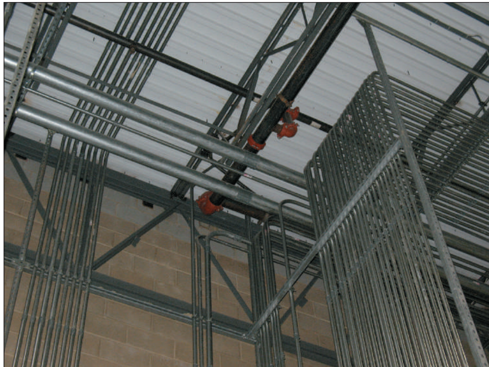
FIGURE 1-1 Electrical metallic tubing (EMT).
