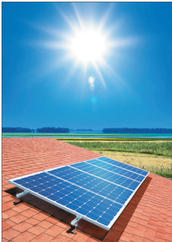
FIGURE 15-2 Solar cell array mounted on a roof.
