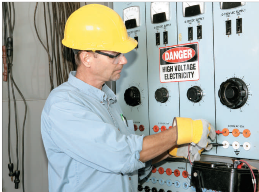
FIGURE 1-11 A maintenance electrician making a measurement.
