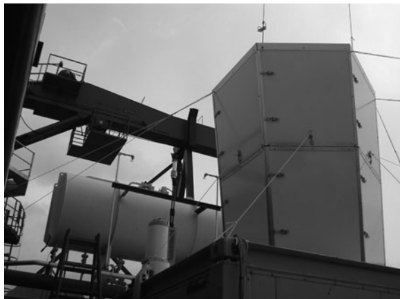
Fig. 1 The ZephIR wind LiDAR in the centre of the image and the AQ500 SoDAR in the front right installed at the Horns Rev platform in 2006
