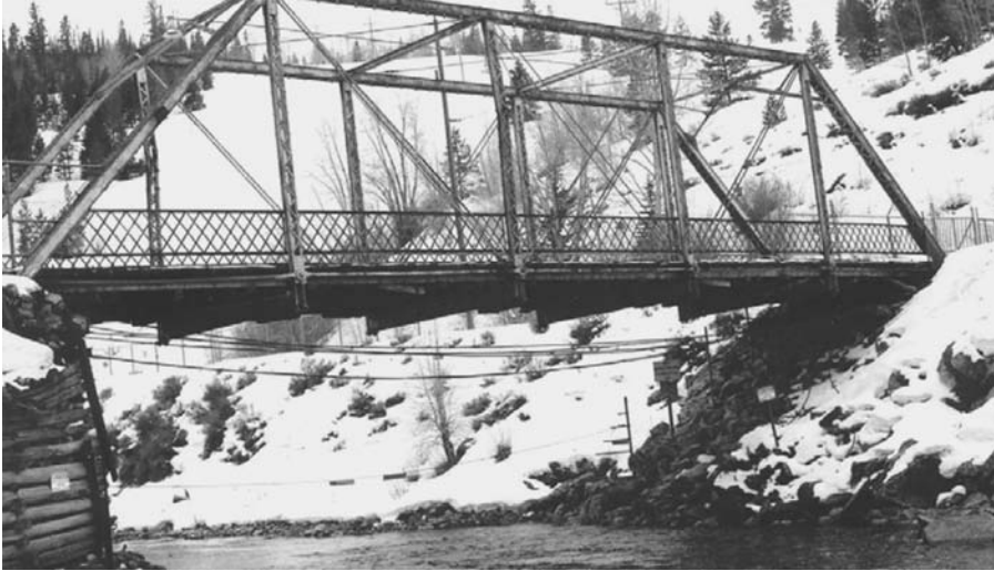
FIGURE 8.3 Blue River Bridge over the Blue River near Silverthorne/Dillon, Colorado. This steel Pratt truss has five bays, with a timber deck on steel stringers. It is believed to have been built approximately 1895 as the Two-Mile Bridge near Breckenridge, Colorado and moved to this site at a later, but unknown, date. Closed to vehicular use, it still serves as a pedestrian crossing of the Blue River. (With permission from ASCE.)
