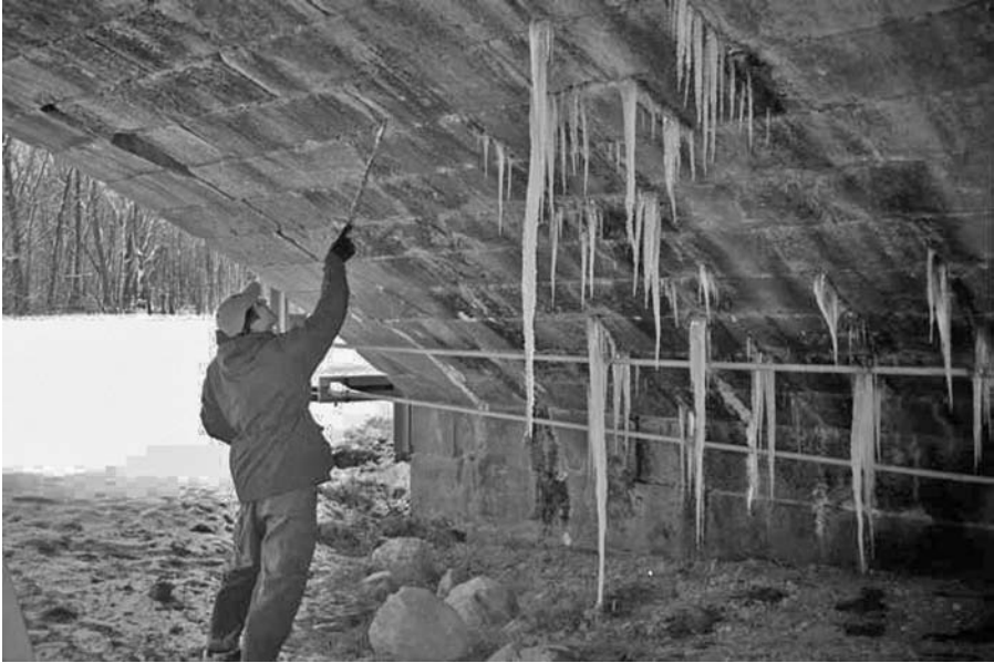
FIGURE 12.9 McMullan & Associates engineer checking ice on arch soffit of the Monocacy Aqueduct.
