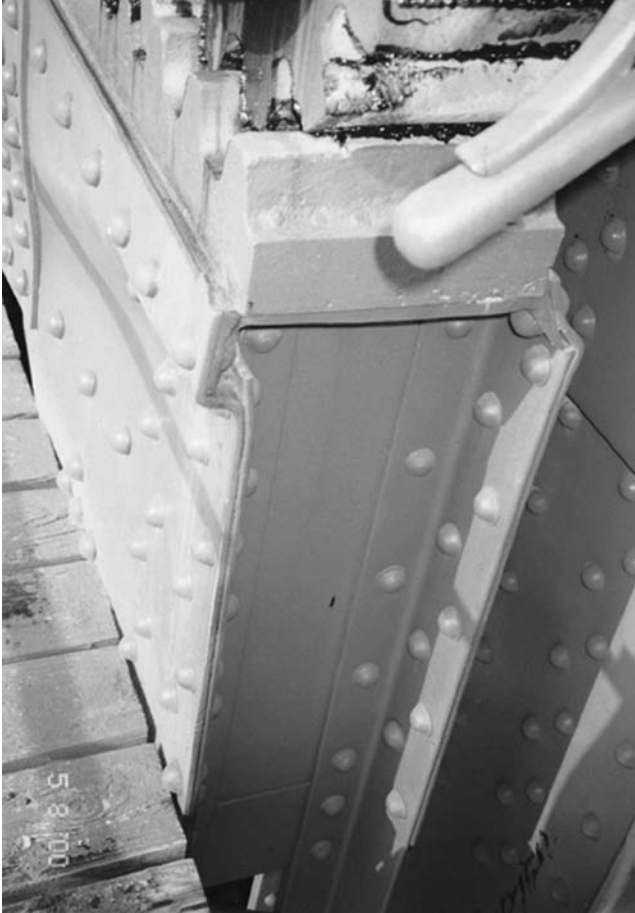
FIGURE 14.9 Fixed Rack, Buckled Track Girder. (Source: Ian Engstrom, Parsons Transportation Group Inc.)
