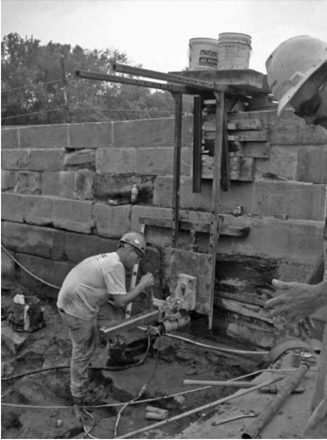
FIGURE 12.21 Drilling hole for reinforcing bars into the parapet at the Monocacy Aqueduct.
