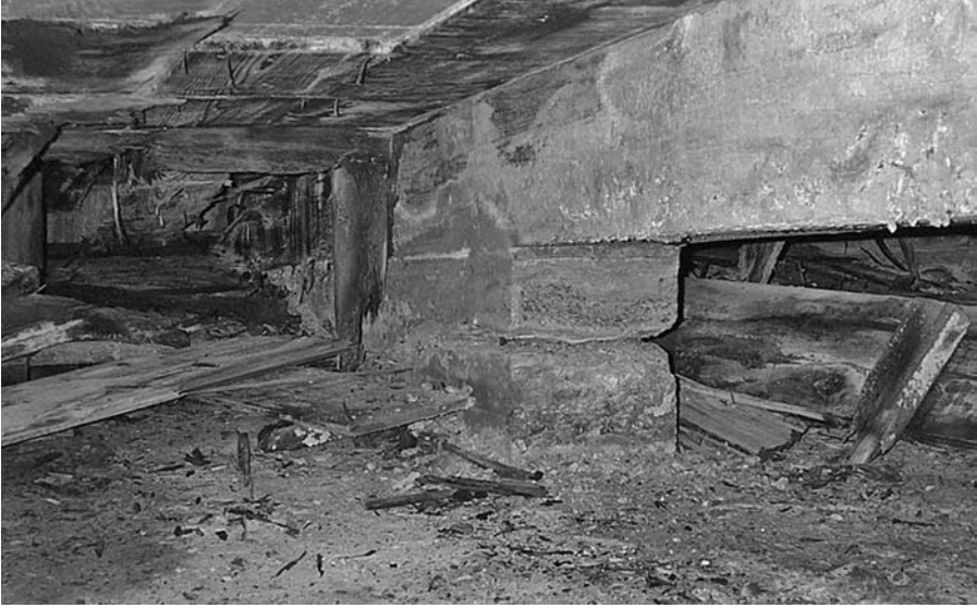
FIGURE 14.6 Deterioration of Arch Superstructure Frame, 2000. (Source: Ian Engstrom, Parsons Transportation Group Inc.)
