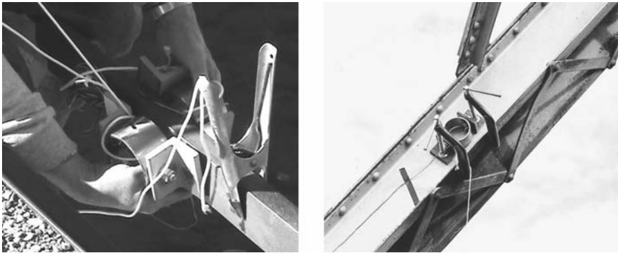
FIGURE 8.18 Strain transducers being installed on bottom-chord eyebars at Prowers Bridge and strain transducer installed on an end diagonal of a portal at Fruita Bridge. Each component has a lanyard attached to it, as a precaution against falling into the river below.
