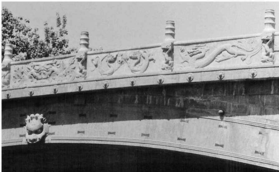
FIGURE 3.7 Close-up view of the An Ji Bridge's new dragon railing panels and posts. Also visible are exterior arch rib fascia details including; cast-iron joint keys, protruding bead highlight strips, and the carved head of a Drinking Water Animal .
