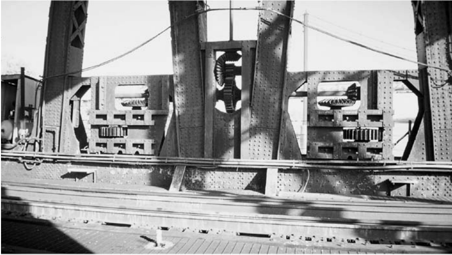
FIGURE 2.19 Span drive intermediate gearing mounted within truss.
