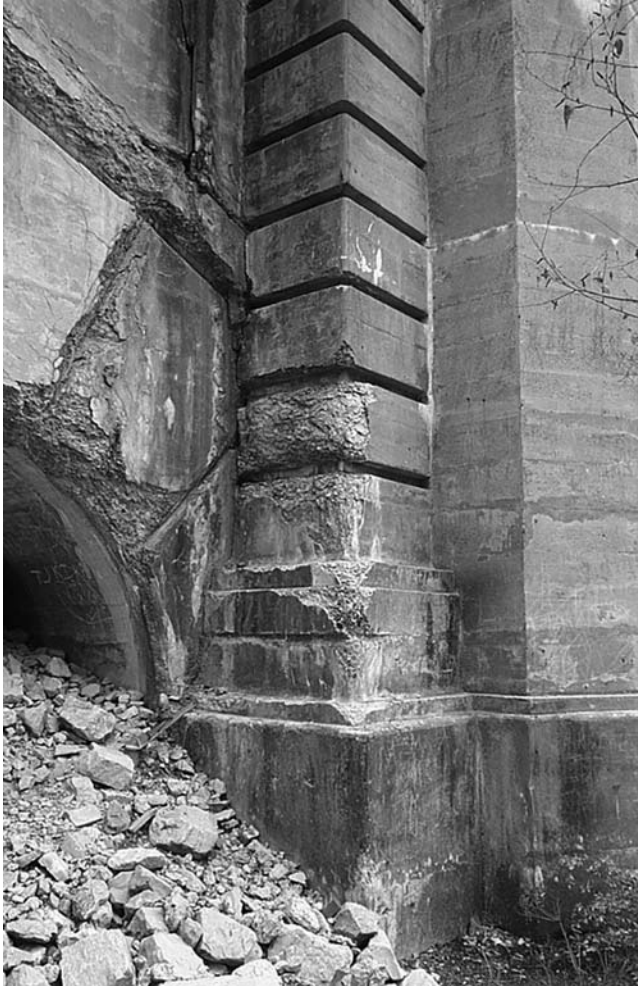
FIGURE 14.5 Deterioration at Abutment 1, 2000. (Source: Ian Engstrom, Parsons Transportation Group Inc.)
