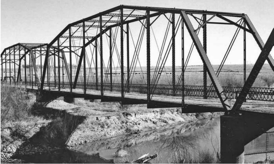
FIGURE 8.5 Prowers Bridge over the Arkansas River, near Lamar, Colorado. The Camelback Pratt through truss span, seen in this photo, was instrumented because it received the greatest wind exposure. It survived a major flood of the Arkansas River in 1921 and served as a highway bridge until its abandonment in 1994 when a nearby replacement bridge was constructed. (With permission from ASCE.)
