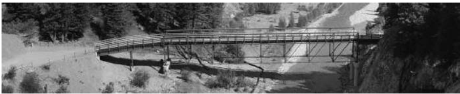
FIGURE 10.3 The Dearborn River deck truss restored. (Source: Montana State Department of Transportation.)
