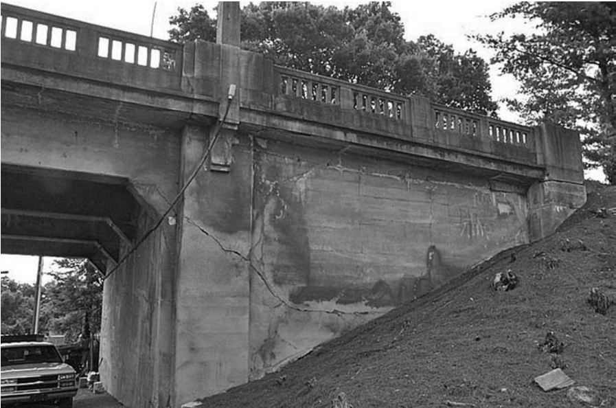
FIGURE 14.7 Deterioration at Abutment 2, 2000. (Source: Ian Engstrom, Parsons Transportation Group Inc.)
