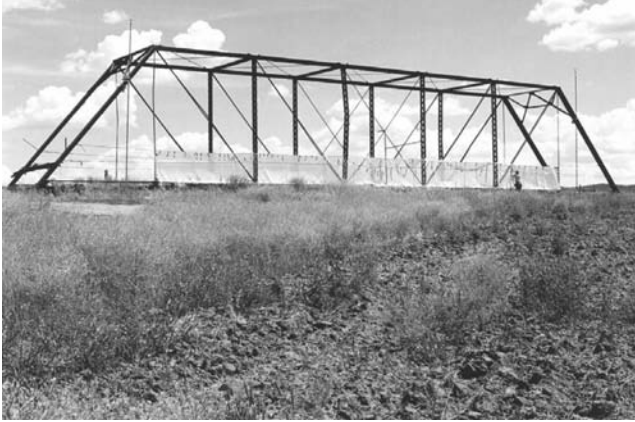
FIGURE 8.20 Overview of sail in place during data collection at Four Mile Bridge.
