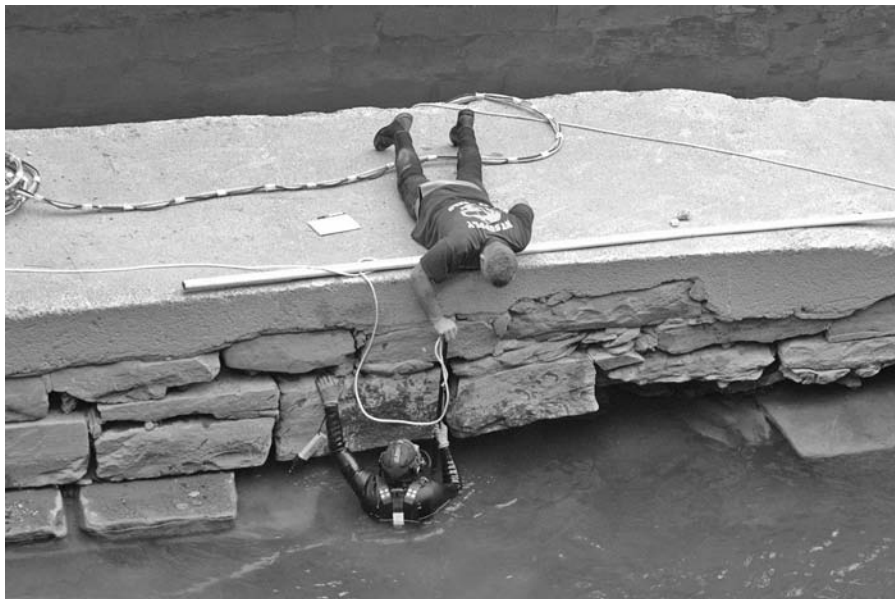
FIGURE 12.16 Underwater inspection of the remains of the west pier at the Catoctin Aqueduct.
