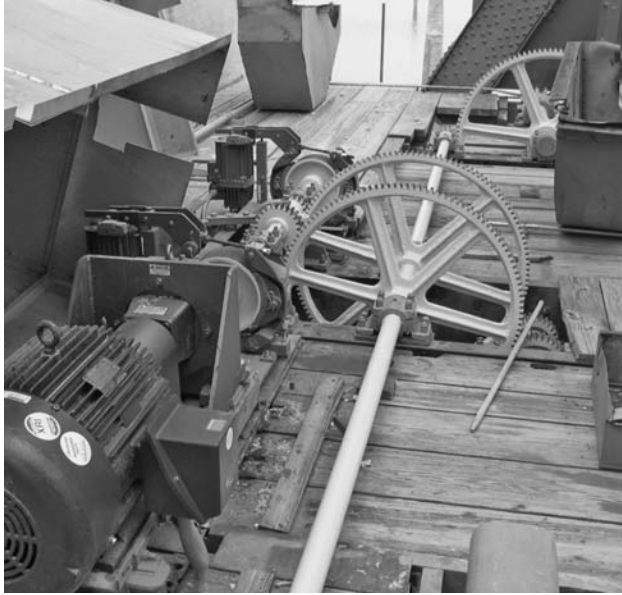
FIGURE 14.14 Mechanical System, 2007. (Source: Ian Engstrom, Parsons Transportation Group Inc.)
