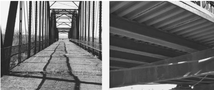
FIGURE 8.6 Prowers Bridge deck. The steel stringers are riveted to the floor beams, suggesting that the stringers are original. However, the corrugated bridge deck is clearly a replacement. Asphalt pavement, now significantly weathered, was installed over the corrugated deck. (With permission from ASCE.)
