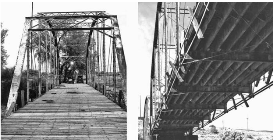
FIGURE 8.2 Fruita Bridge deck. The deck timbers are spiked to timber stringers, which bear on steel floor beams. The deck is discontinuous in that there are gaps between the deck timbers. The short vertical timbers are the remnants of the former wood rail.
