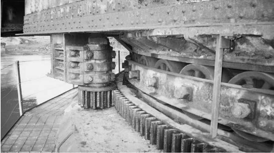
FIGURE 2.16 Rim bearing assembly and span drive pinion.
