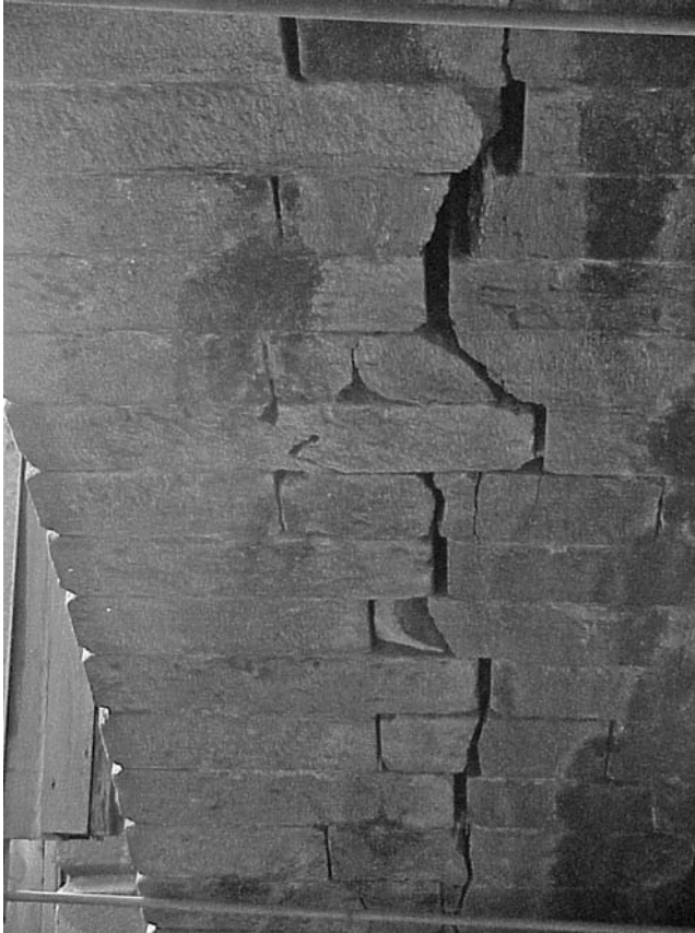
FIGURE 12.19 Longitudinal cracks in one of the Monocacy Aqueduct's arch barrels.
