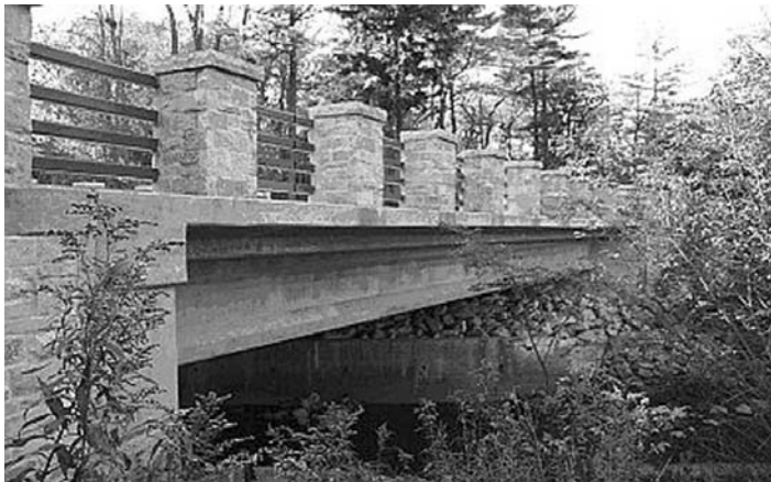
FIGURE 4.6 In an effort to match the original design and materials, the new Oak Creek Bridge (P40-559) featured steel railings embedded in veneered posts and stone-veneered abutments. However, the modern styling of the multiple railings and posts contrasts with the simplicity of its historic, rustic design. (Photo by author.)
