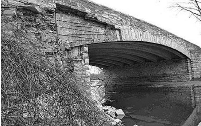
FIGURE 4.8 The Milwaukee River Bridge (B40-647) displays deteriorated abutment walls and spalling stonework. With a sufficiency rating of 34.7, it is scheduled for replacement in 2008. (Photo by author.)
