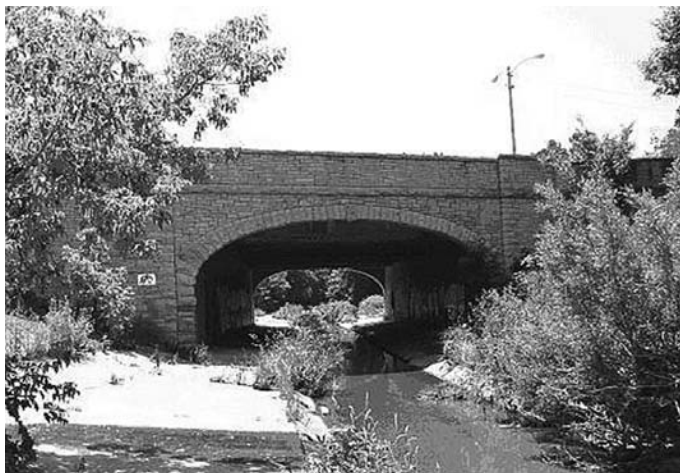
FIGURE 4.5 The West Forest Home Avenue Bridge (B40-979) is a 1931 concrete T-beam bridge with a stone-faced headwall that features a segmental arch opening. Its handcrafted, rock-faced, limestone parapet walls feature a random ashlar pattern. (Photo by author.)
