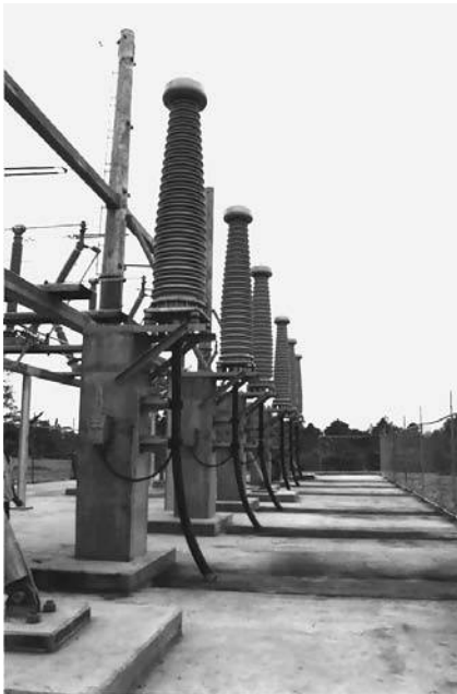
FIGURE 14-96 Terminations mounted on concrete risers.
