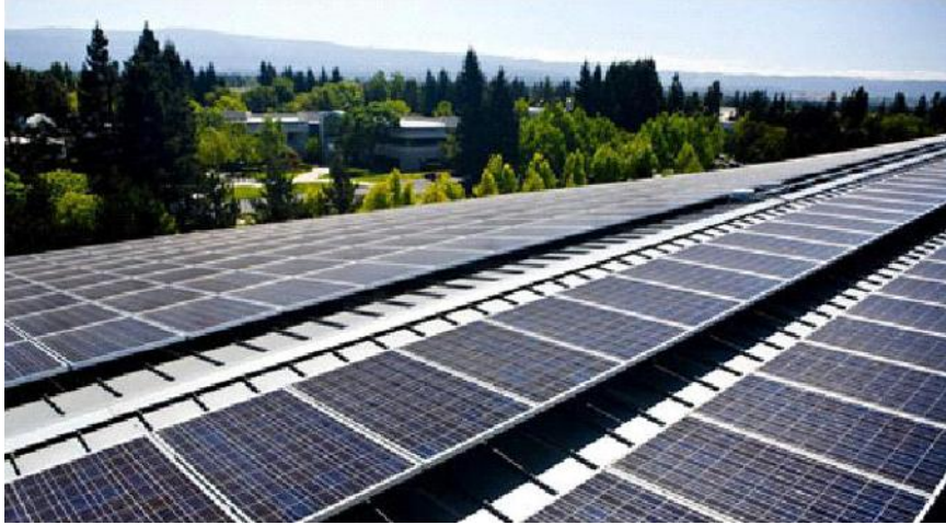
Figure A.3 A view of solar collectors [2].
