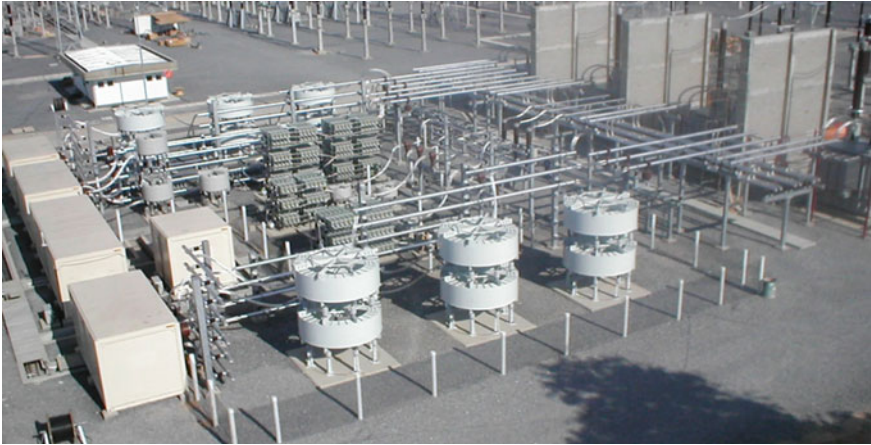
Fig. 3.53 SVC plant \pm 250 Mvar ( Source Siemens AG)
