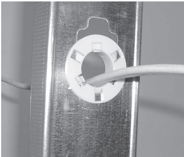
Figure 15-17. Nonmetallic-sheathed cable installed through metal framing.
