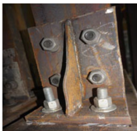
(k) Bending deformation of the stiffening rib
