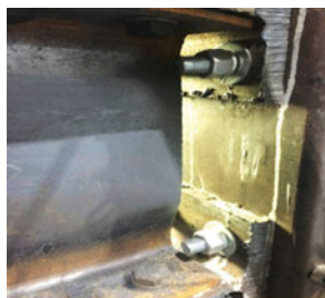
(j) Bending deformation of the steel beam web
