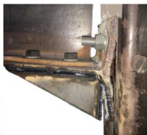
(l) Cracking of the vertical weld
