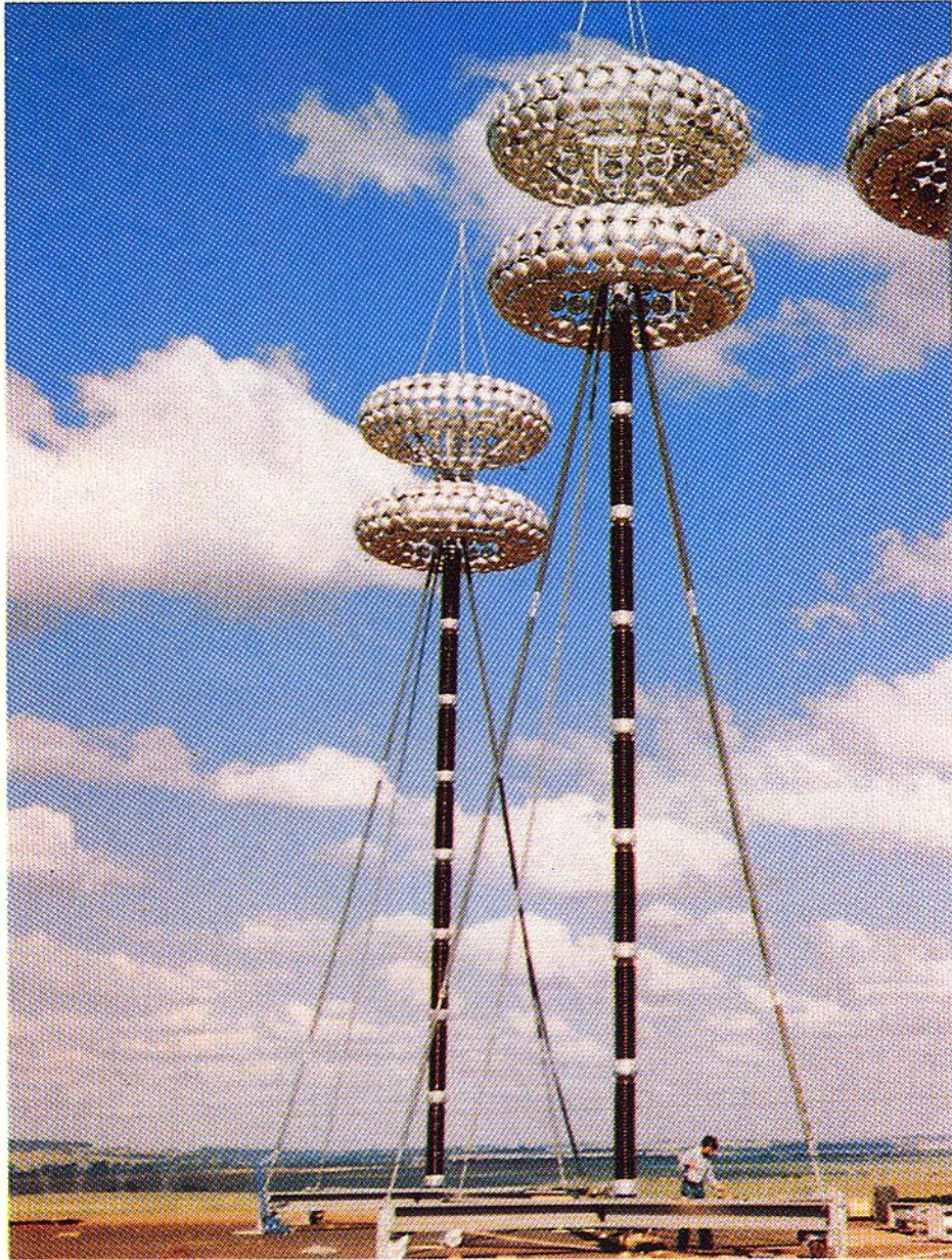
Large outdoor impulse voltage dividers, damped capacitive type with large top electrode for ultra-high switching impulse voltages
