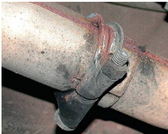
Figure 1.71 Corrosion on an exhaust joint
