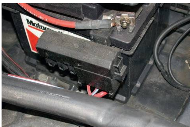
Figure 3.20 Heavy cable from the battery
