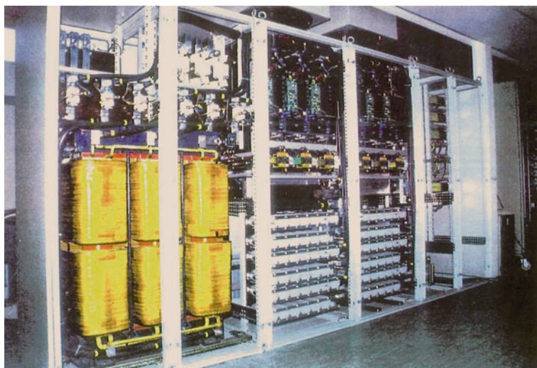
Fig. 10.46 500kVA 12-pulse current source converter
