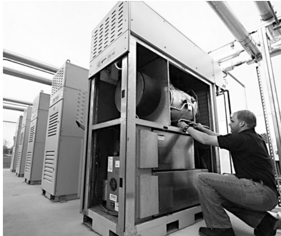
Fig. 8.1 Installation of several 65 kW microturbines
