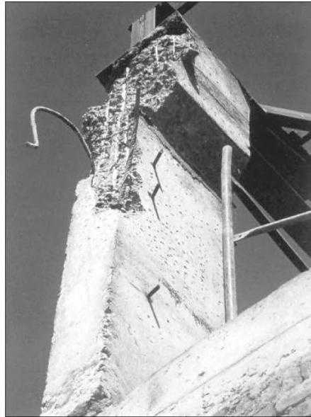
Figure 1.3 Column where edge beam has broken off.
