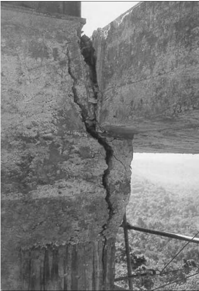
Figure 1.2 Edge beam starting to separate from column.
