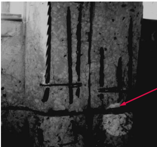
Figure 8.17 Spalling of mullions. (Courtesy of Poul Beckmann.)
