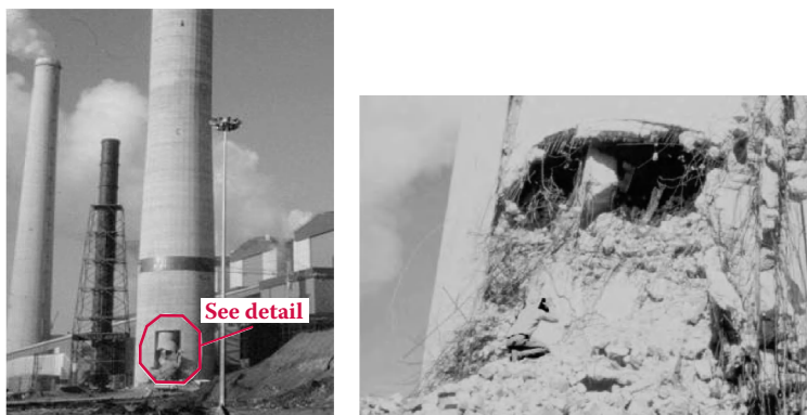
Detail: Close up of debris
