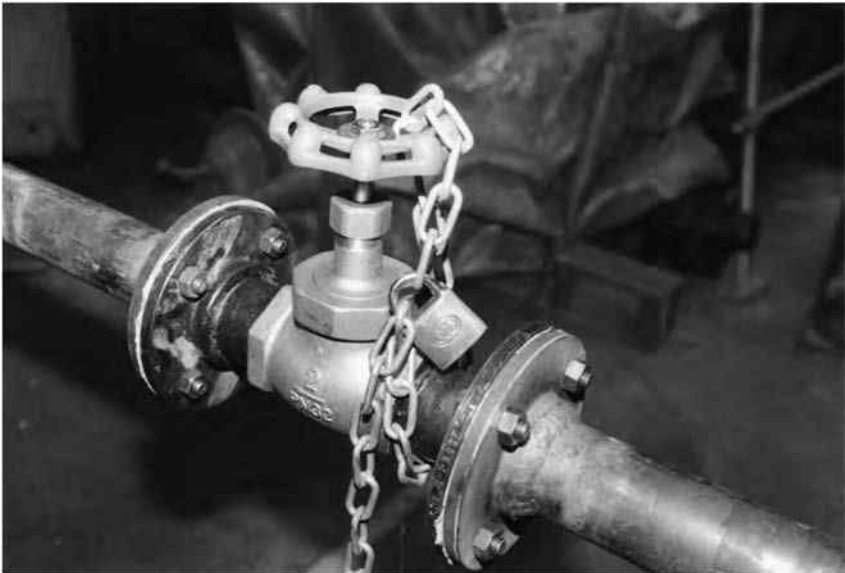
Figure 14.1 Examples of locking off (a) an electrical switch and (b) a valve.
