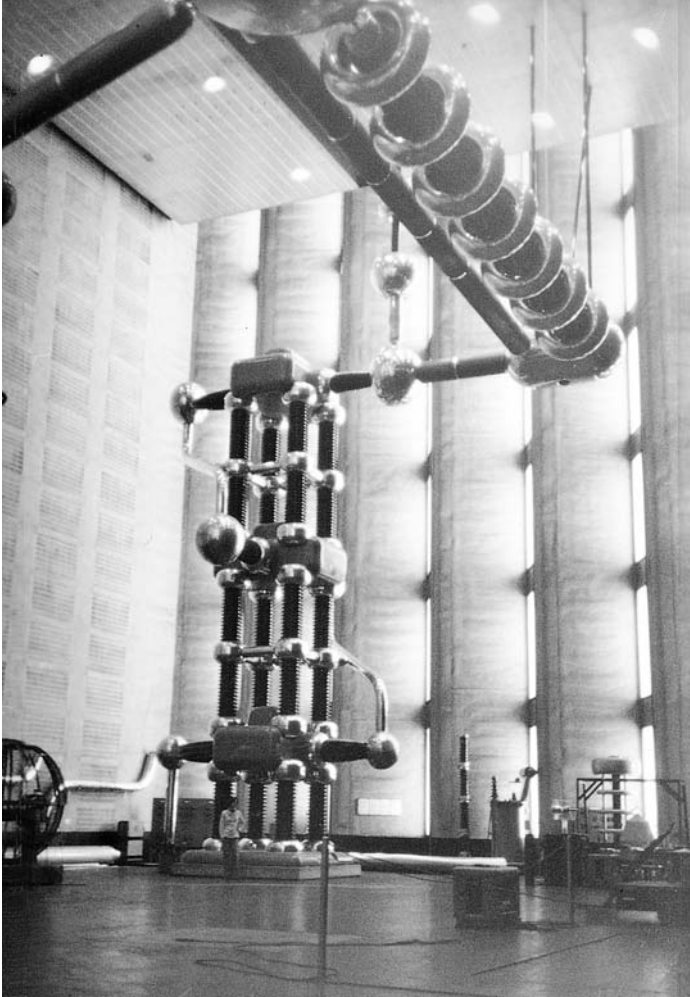
Figure 2.14 Testing transformer for 1200 kV r.m.s. comprising three single unit transformers according to Fig. 2.13, with metallic tanks and bushings (High Voltage Laboratory, Technical University of Munich, Germany). (Note. Suspended at ceiling and connected with transformer is a selenium-type rectifier with a reverse voltage of 3.4 MV, see ref. 5.)
