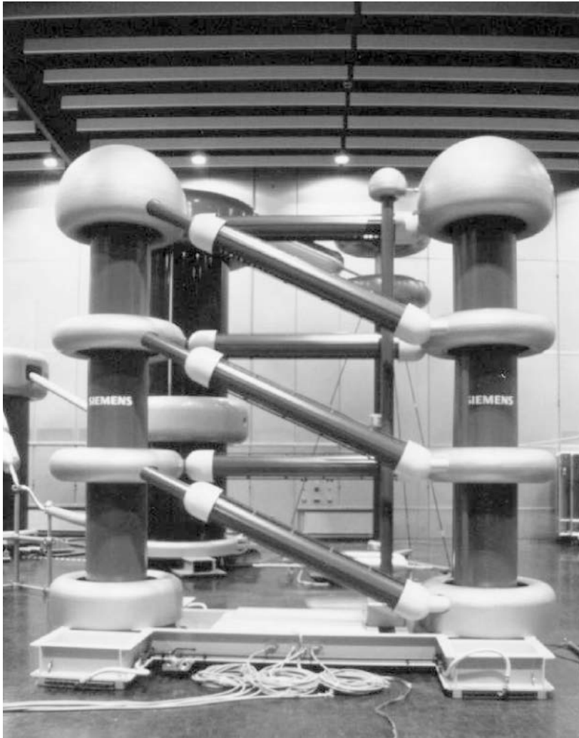
Figure 2.5 A Cockcroft–Walton d.c. generator for voltages up to 900 kV/10 mA with fast polarity reversal at ETH Zurich (courtesy HIGH VOLT, Dresden, Germany)
